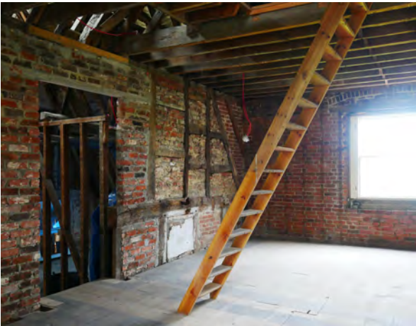
68. Victorian southern cross-wing. The NE corner of room shows the original external southern wall of the three-bay building. The original end wallplate has been served losing the west side. Evidence of a former windows. Brick infills not maintained properly. Evidence of 2 stages of change to the roof.
