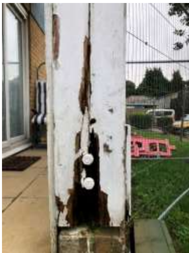
Photograph One - rot to base of timber column
