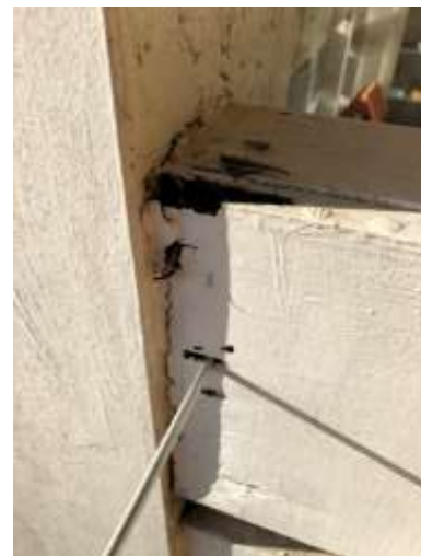
Photograph Two - rot to balustrade
