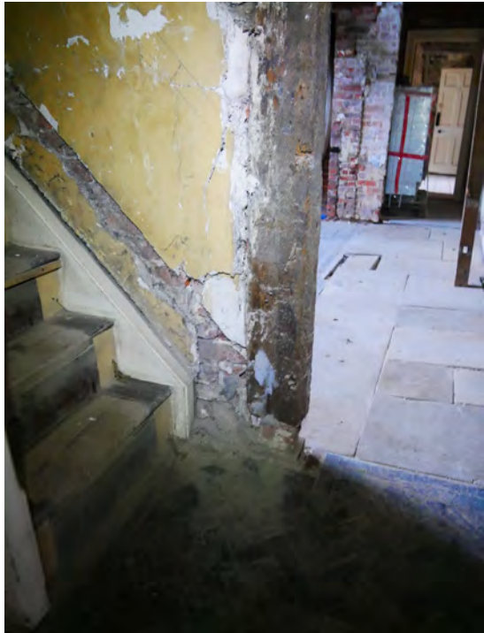
28.Edge of G13 Stair with post to door leading into G10. Evidence of wattle and daub to rear of wall of G9. The base post has eroded at the base requiring brick underbuilding.
