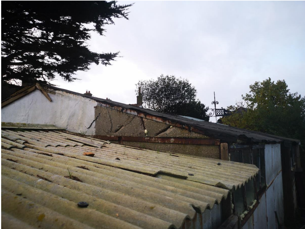
Structural damage to the supporting wall on the North East facing side
