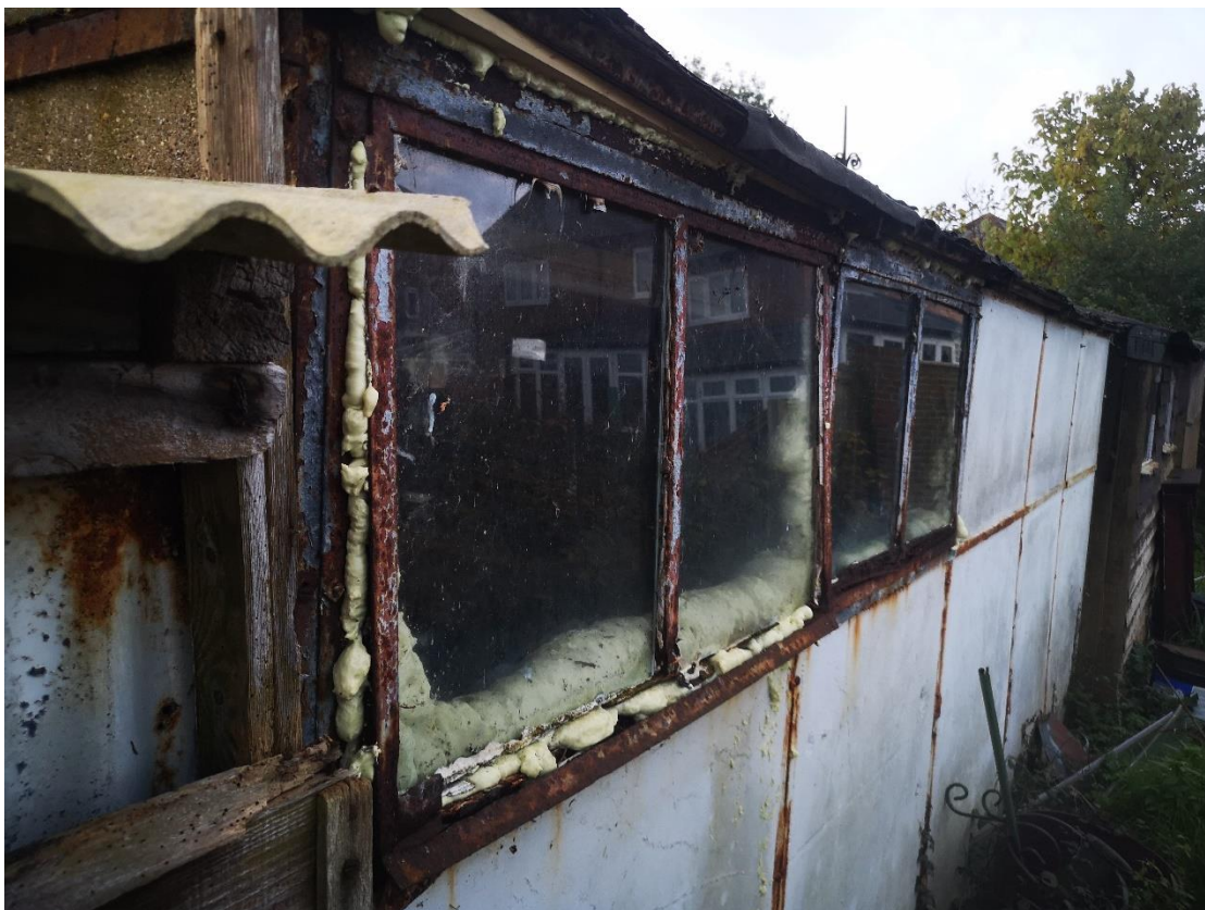
Decay window frames and structure which has been filled with expanding foam by previous owners
