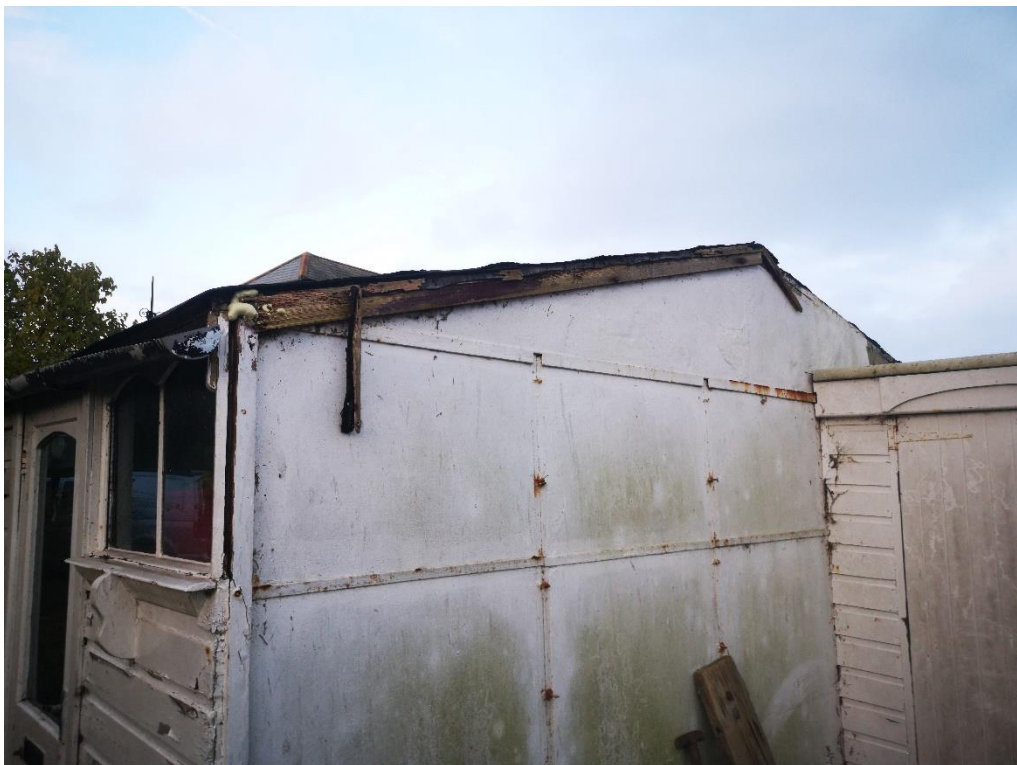
Decay of the roof structure
