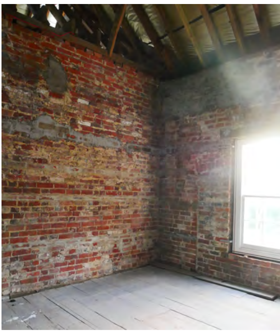
64. FF5 SW - Noteable mark/cambered brick lintel for a bay. Sth wall also shows signs of wall plate increase with later Victorian cross wing added. Evidence of old cement repairs.
