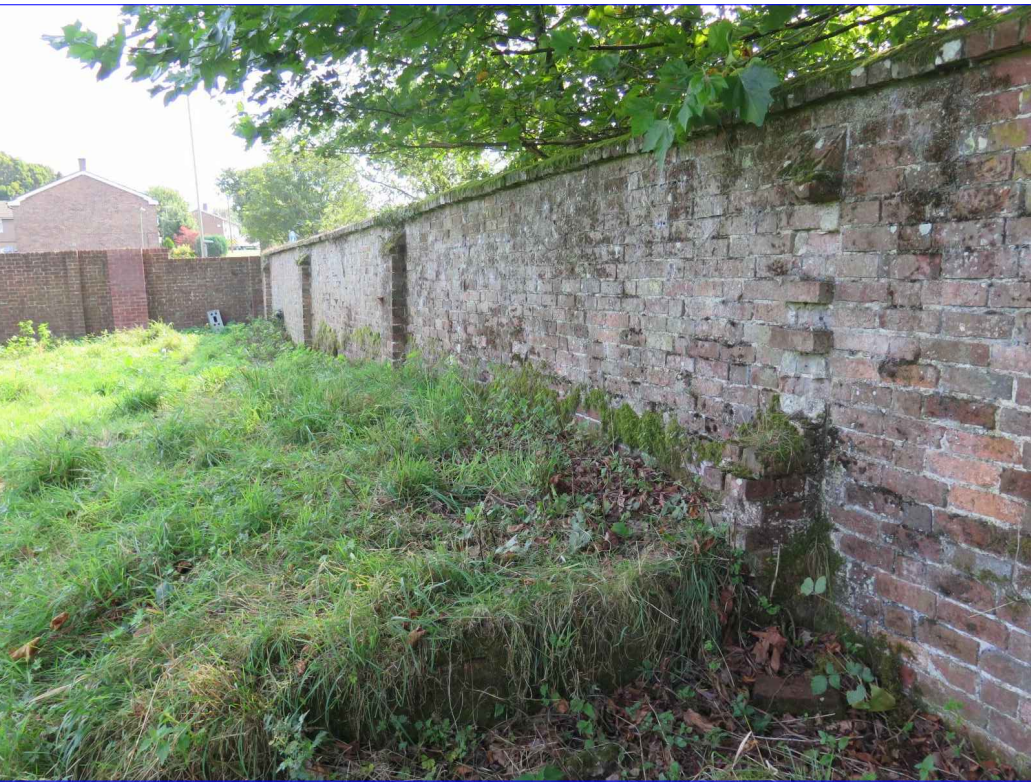
1 — Collapsed piers to be rebuilt as shown on drg 1100
