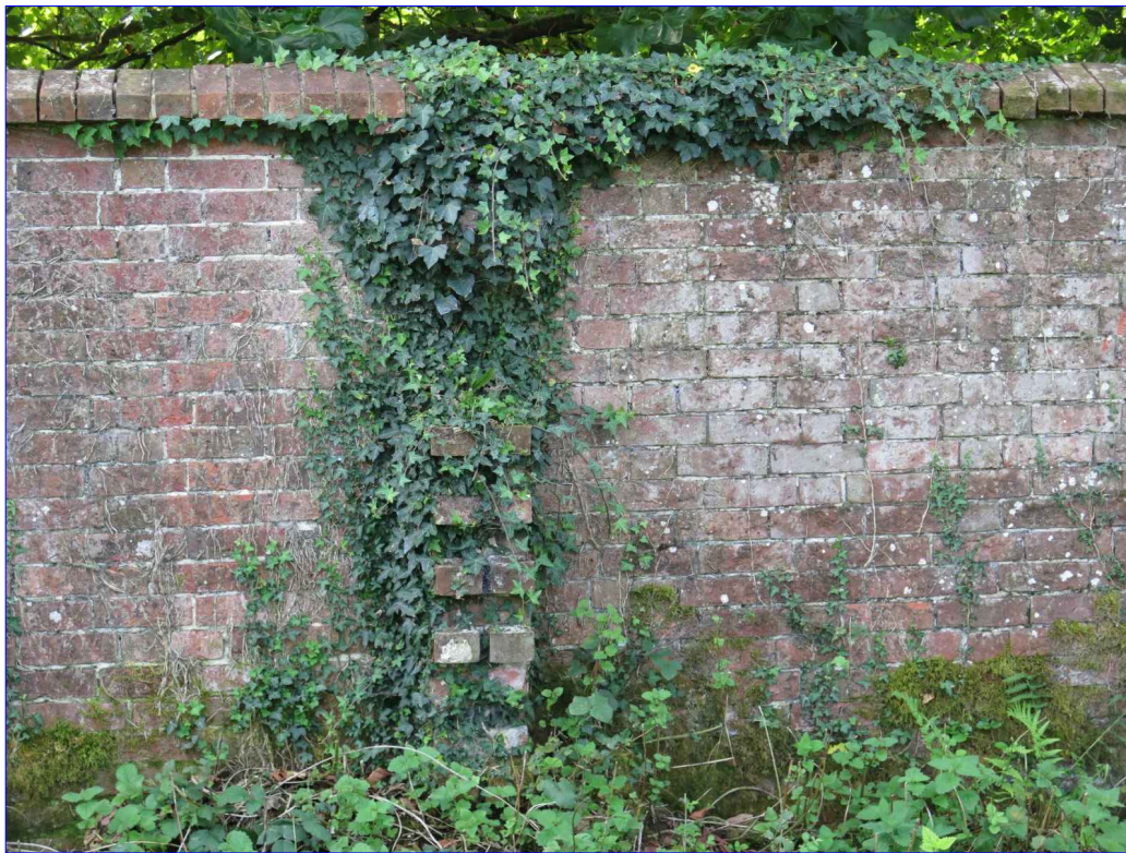
2 — Ivy to be removed from wall and piers
