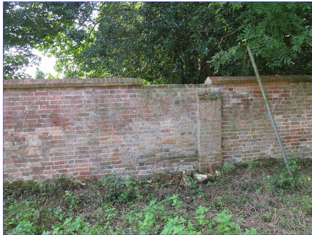
3 — Missing copings to be replaced with new matching and report all loose coping joints.
