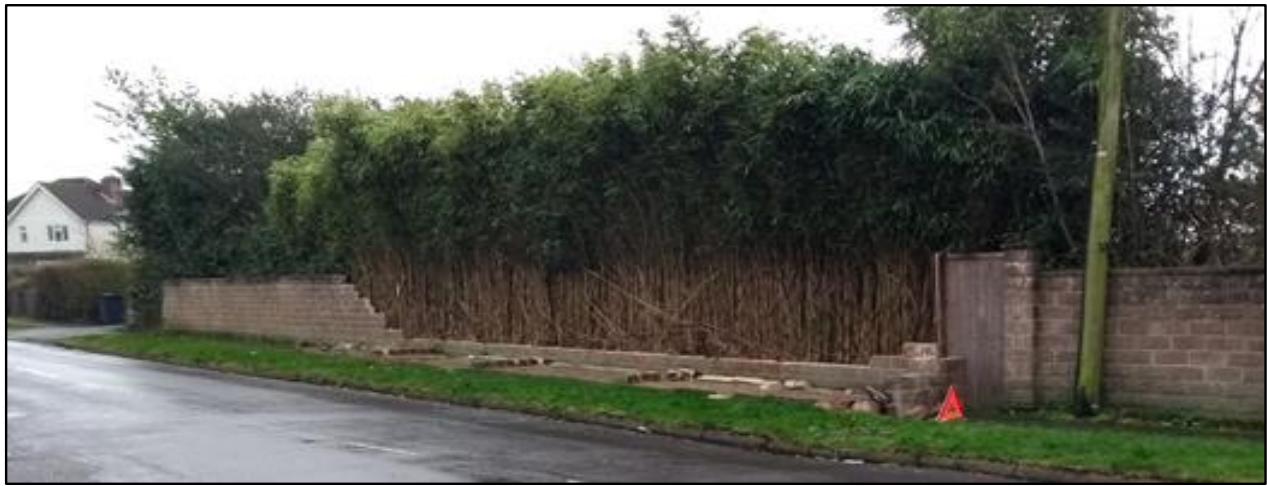
Current state of boundary wall
