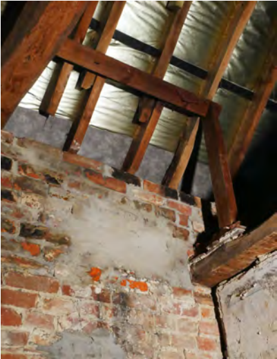
49. View of NW corner revealing parting of west face from inner north wall and raised height. Evidence of past cement repairs.
