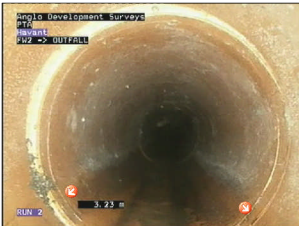
Photo: 3_3_11_A.JPG 3.2m, Crack, circumferential at joint, from 12 to 12 o'clock
