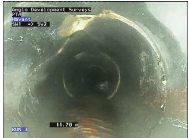
Photo: 4_4_19_A.JPG 11.7m, Broken pipe, from 12 to 12 o'clock, Start
