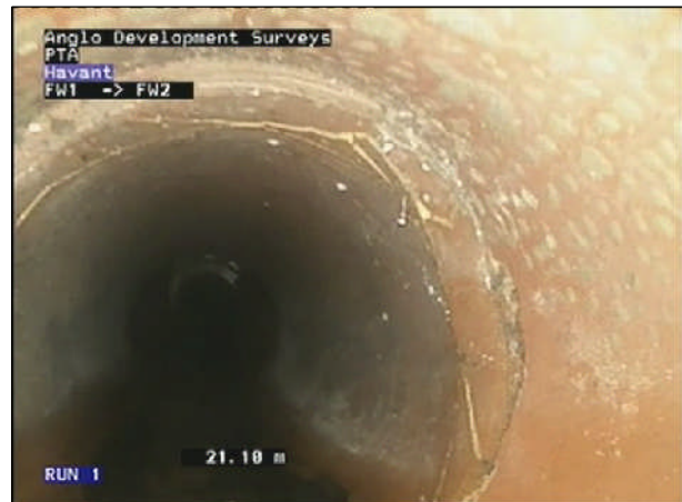
Photo: 1_1_7_A.JPG 21.1m, Cracks, multiple at joint, from 12 to 12 o'clock
