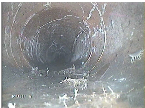
Photo: 7_7_35_A.JPG 0.3m, Fracture, multiple, from 12 to 12 o'clock, Start
