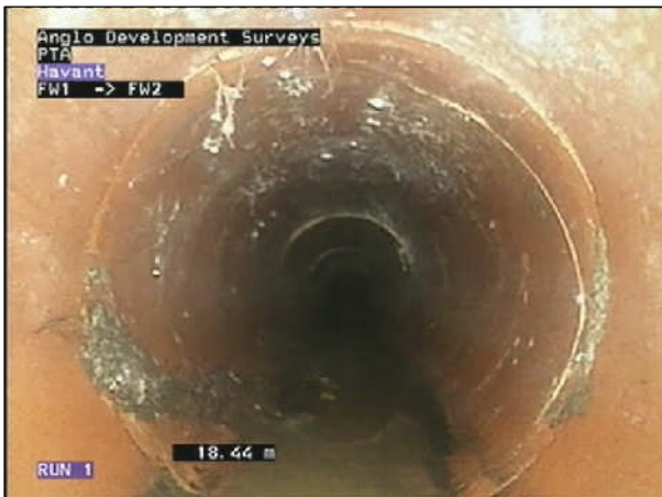
Photo: 1_1_5_A.JPG 18.4m, Crack, circumferential at joint, from 9 to 4 o'clock
