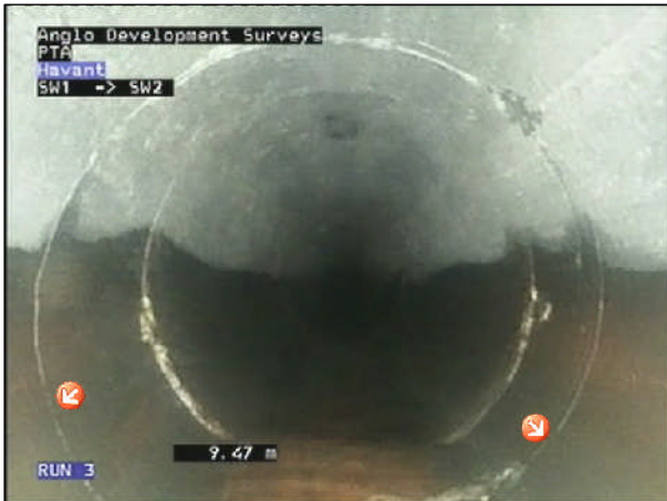
Photo: 4_4_18_A.JPG 9.4m, Crack, circumferential, from 12 to 12 o'clock
