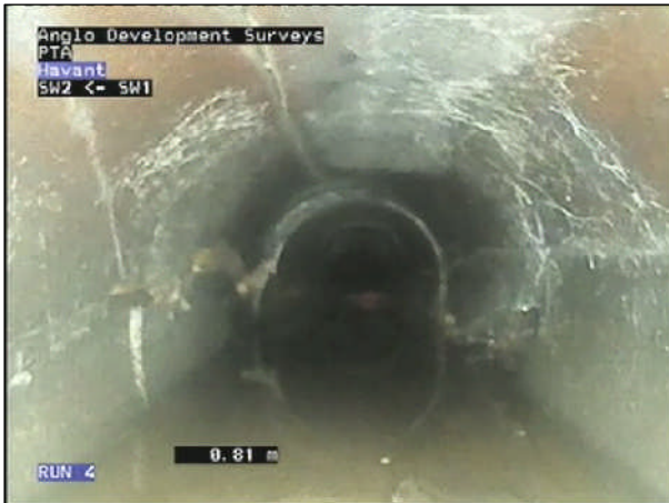
Photo: 5_5_24_A.JPG 0.8m, Broken pipe, from 12 to 12 o'clock, Start
