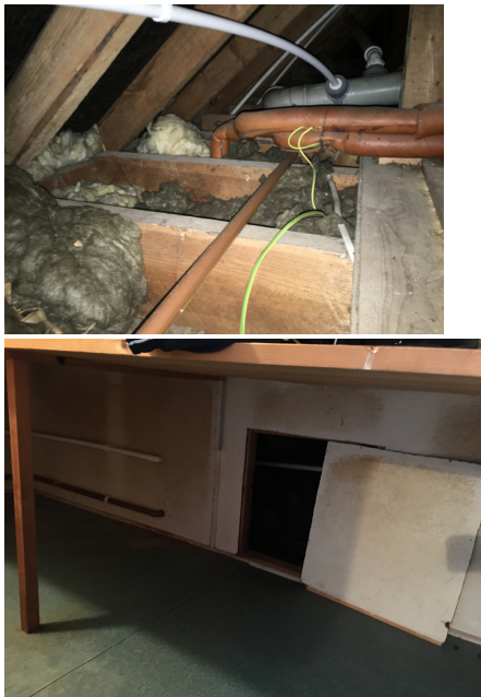
Figure 5 & 6. Voids present within the main house
