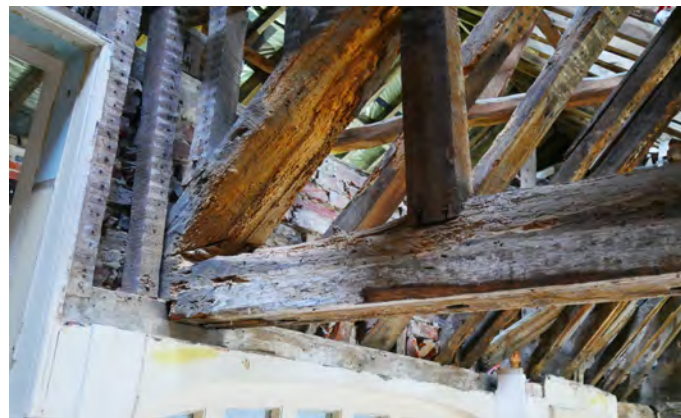
54. Closer view of the missing post. The wall plate has been altered in this area. There is evidence of a partition / door in this location.
