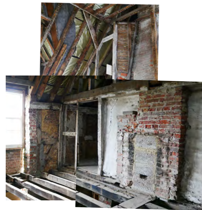
57. The East wall plate, rail and side girt was cut for the late Victorian Bay. Scar marks can be seen for the former ensuite partition. The timber in this area was disintegrating & brickwork collapsing. A former window to FF10 was also uncovered as well the doorway to the garrett above. Modern blocks to fireplace.
