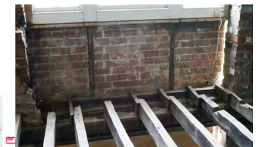
59. The Victorian bay is a mere 'bolt on', not tied in correctly to the main frame. Extensions to floor joists are the method of support. Also concealed with modern coverings.
