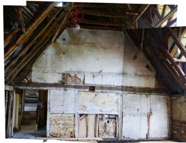
56. An amalgamated photograph showing the inner north wall plus former garret above. Evidence remains for the former spine position, the scar mark for the modern partition and two different ceiling heights. Daub panels have been repaired.
