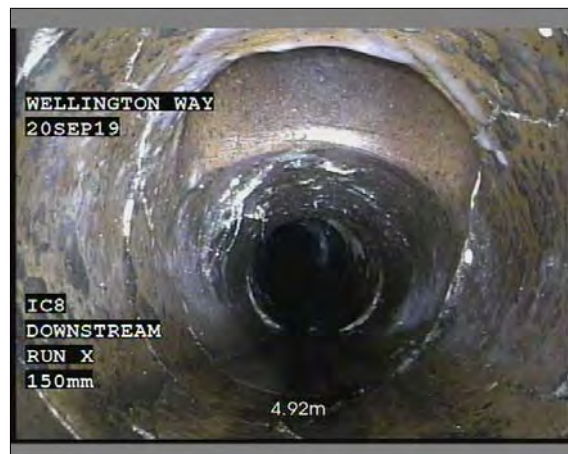
Photo: 004.JPG, VCR No.: 00002 4.92m, Fractures, multiple, from 12 to 12 o'clock
