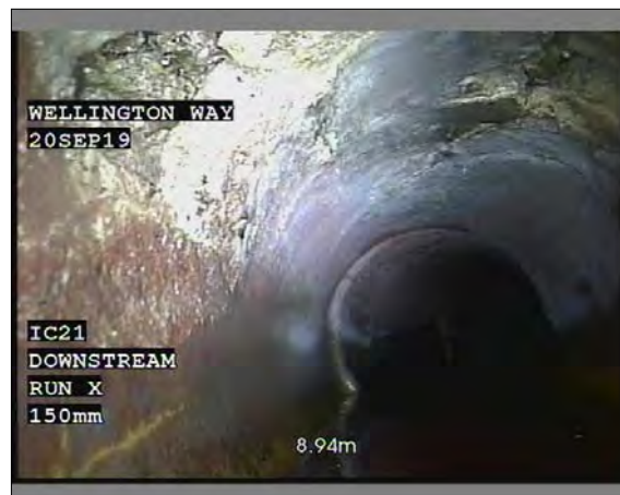
Photo: 012.JPG, VCR No.: 00004 8.94m, Hole in sewer, at 10 o'clock
