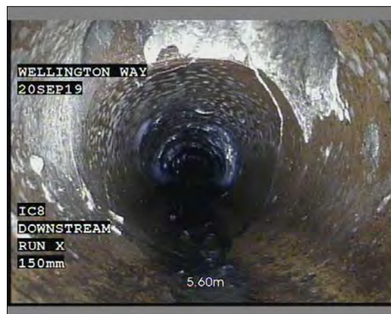
Photo: 006.JPG, VCR No.: 00002 5.6m, Crack, circumferential, from 12 to 12 o'clock
