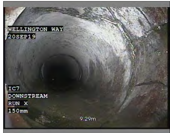
Photo: 002.JPG, VCR No.: 00001 9.29m, Fracture, multiple at joint, from 12 to 12 o'clock
