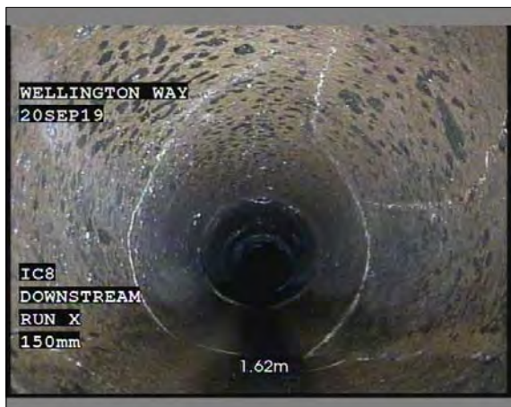
Photo: 003.JPG, VCR No.: 00002 1.62m, Cracks, multiple, from 12 to 12 o'clock
