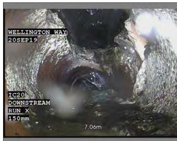
Photo: 009.JPG, VCR No.: 00003 7.06m, Encrustation, heavy, from 4 to 7 o'clock, 30% cross-sectional area loss, Start
