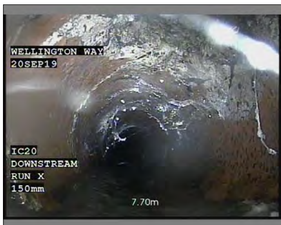
Photo: 010.JPG, VCR No.: 00003 7.7m, Hole in sewer, from 10 to 2 o'clock
