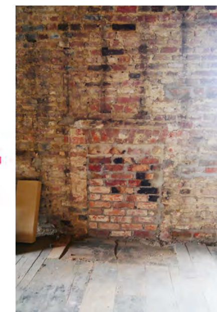
96. Fireplace to FF16 blocked up. Hearth slab cracked.
