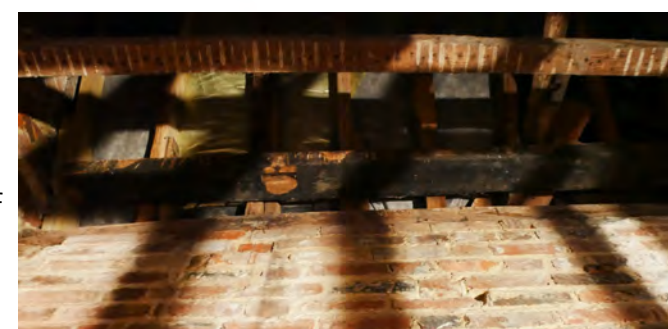
97. Fire damage to timbers that have been reused above to FF16 and FF17.
