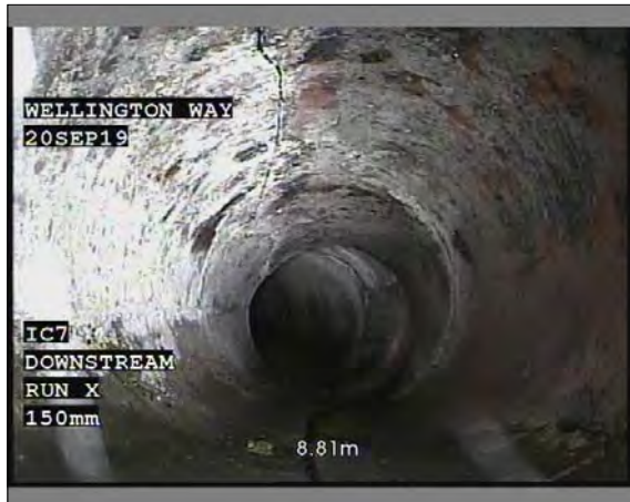
Photo: 001.JPG, VCR No.: 00001 8.81m, Fractures, multiple, from 12 to 12 o'clock
