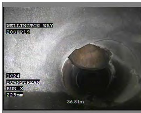
Photo: 015.JPG, VCR No.: 00005 36.81m, Connection, at 12 o'clock, 150mm diameter, 40mm intruding
