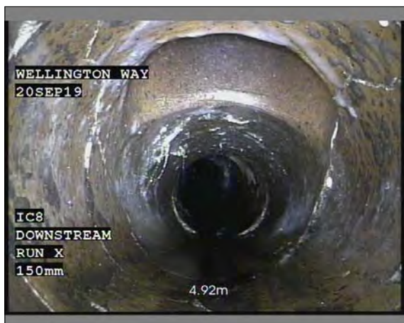
Photo: 005.JPG, VCR No.: 00002 4.92m, Junction, defective, at 12 o'clock, 150mm diameter
