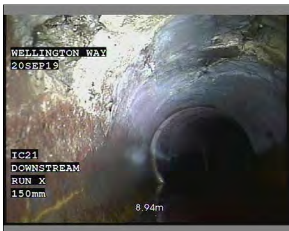
Photo: 013.JPG, VCR No.: 00004 8.94m, Cracks, multiple, from 9 to 3 o'clock
