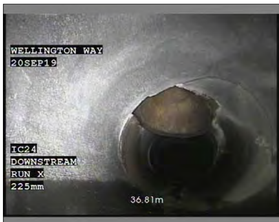
Photo: 014.JPG, VCR No.: 00005 36.81m, Cracks, multiple, from 12 to 12 o'clock
