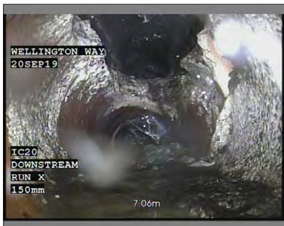
Photo: 008.JPG, VCR No.: 00003 7.06m, Hole in sewer, from 10 to 2 o'clock
