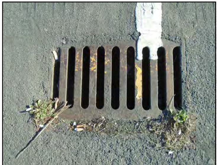
GULLY 9 UNABLE TO LIFT
