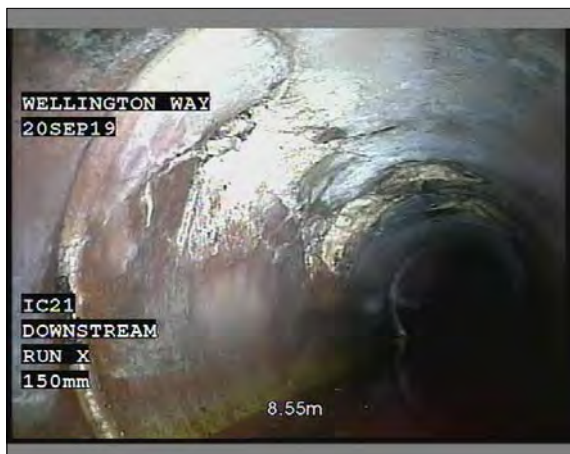
Photo: 011.JPG, VCR No.: 00004 8.55m, Hole in sewer, at 10 o'clock
