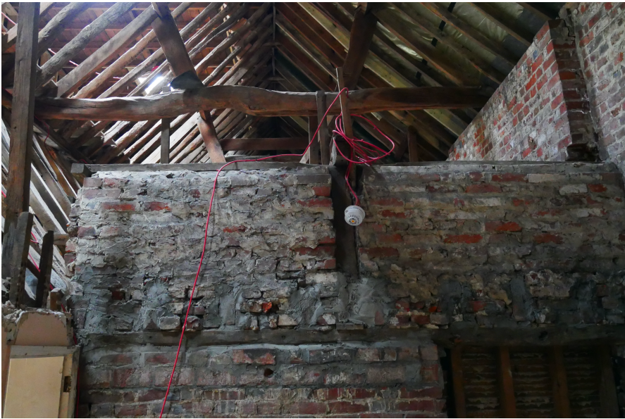
78. South wall to FF12 shows evidence of intruded stair bay. The roof struture is basic in this position, unlike the roof over FF5.
