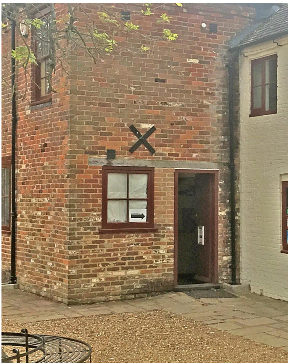
Fig 5. Existing north return elevation of Regency Farmhouse, indicating modern brickwork between door and window, existing full width timber lintel, vent grille above, and inadequate signage.
