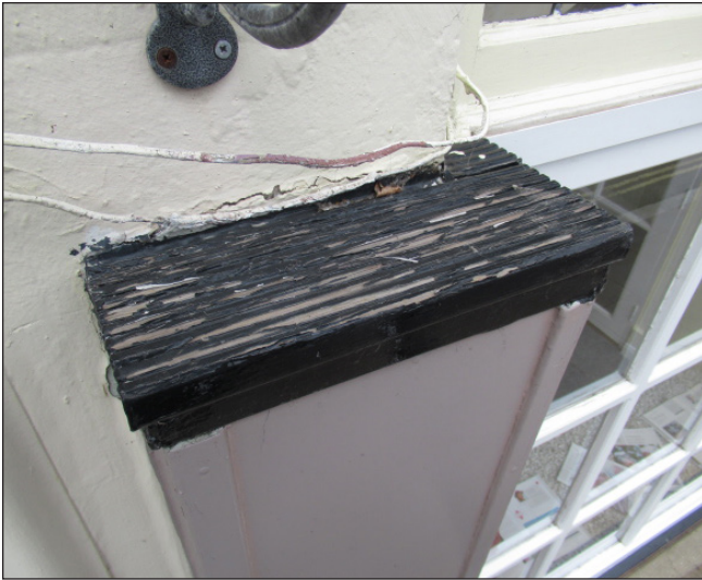
Top columns are peeling Will require repainting
