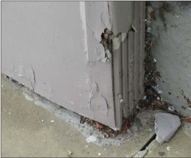
Woodwork rotten Will require repairing
