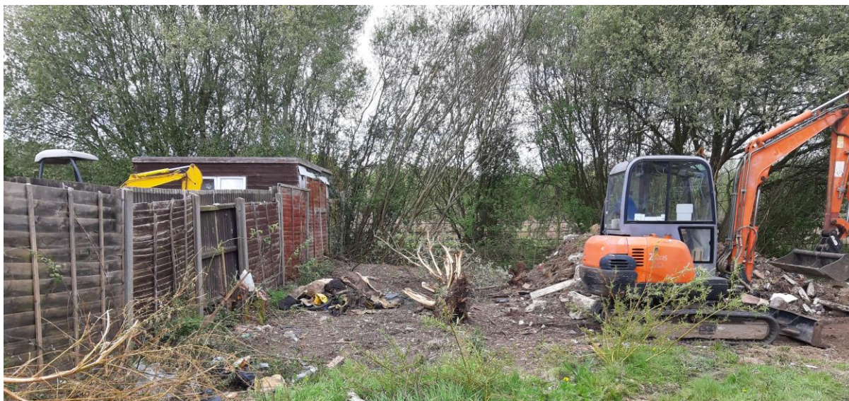
Photo 1: Building material being stored on site
