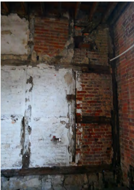
12. NE Corner of room. Diagonal brace has partly deteriorated. Lime wash to former external wall.
