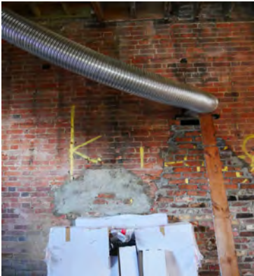
13. Position of former fire place. To be replaced.
