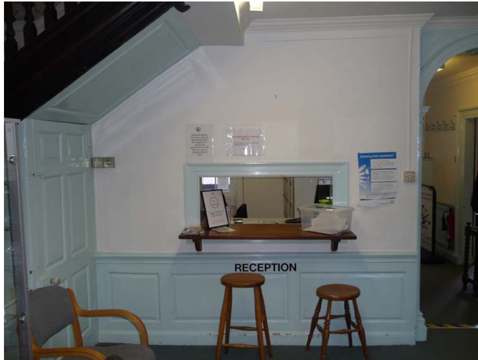
Modern reception window to be blocked in to reinstate wall.
