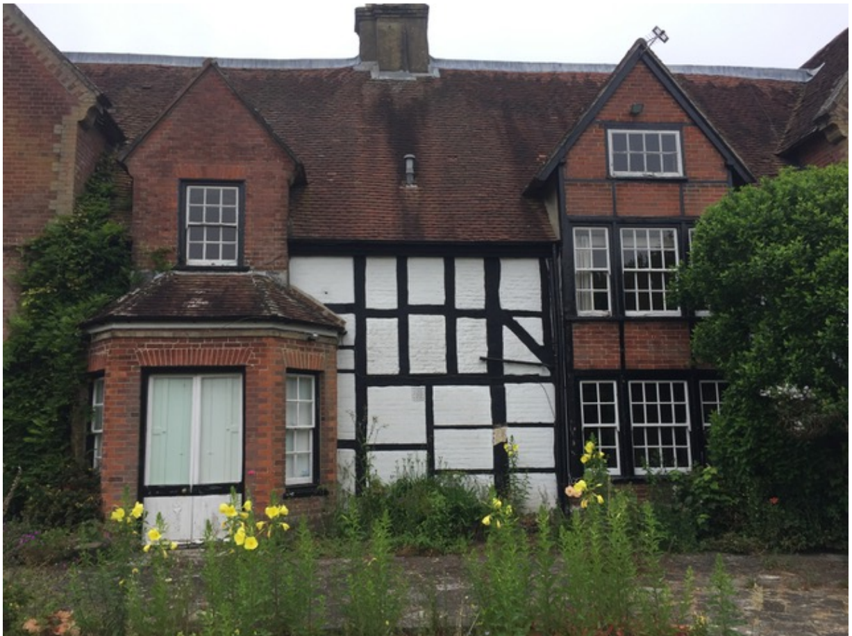
Before with roof on showing signs of failure of flashing, bonnets and delamination of tiles
