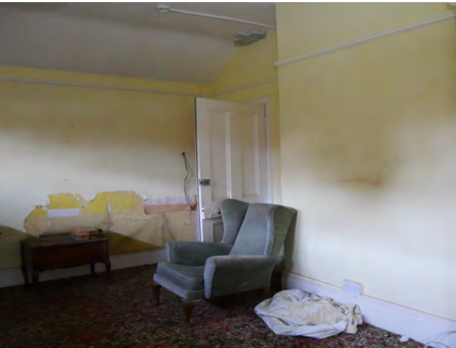
44. Blocked up fireplace to G18, west inner wall with chimney breast obscuring a Victorian window.
