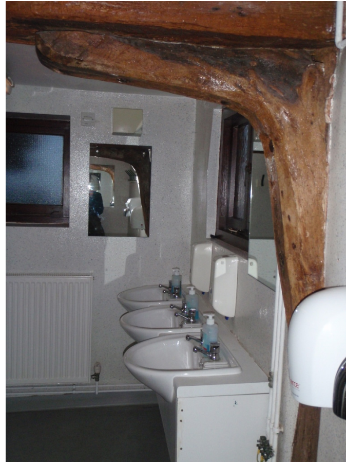
12. Female toilets to be refurbished.
