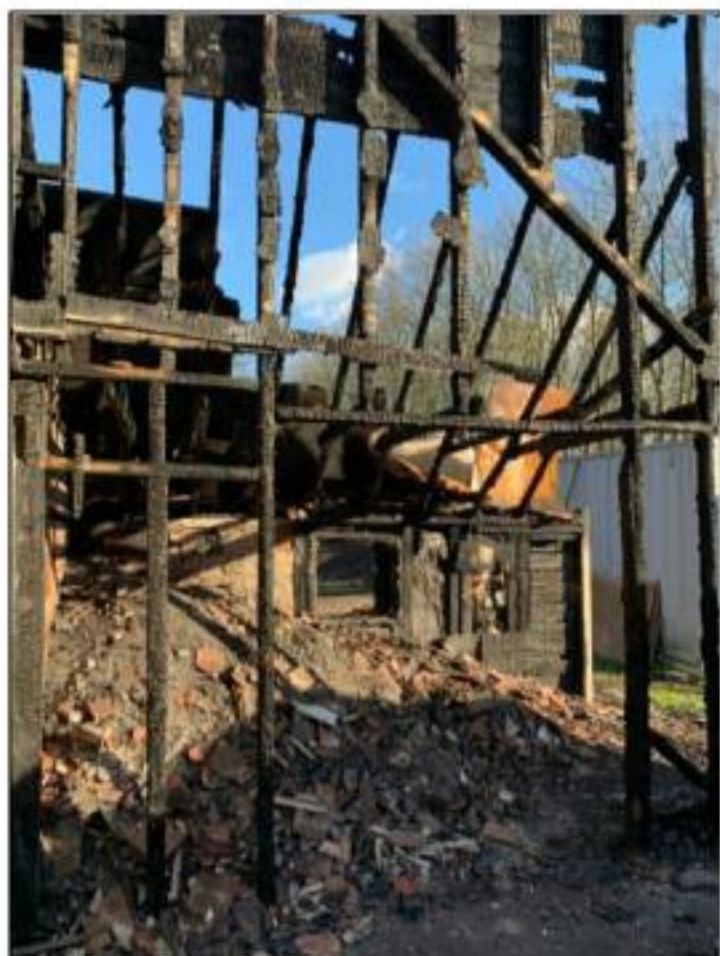
Figure 23: The cottages after the devastating fire (Jan, 2019)
