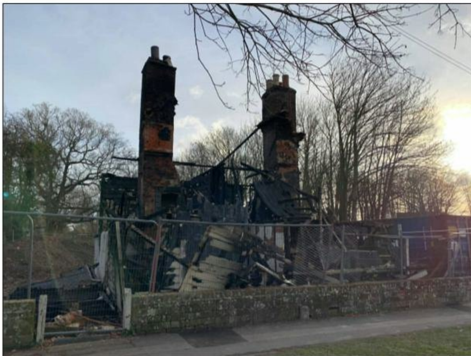
Figure 22: The cottages after the devastating fire (Jan, 2019)
