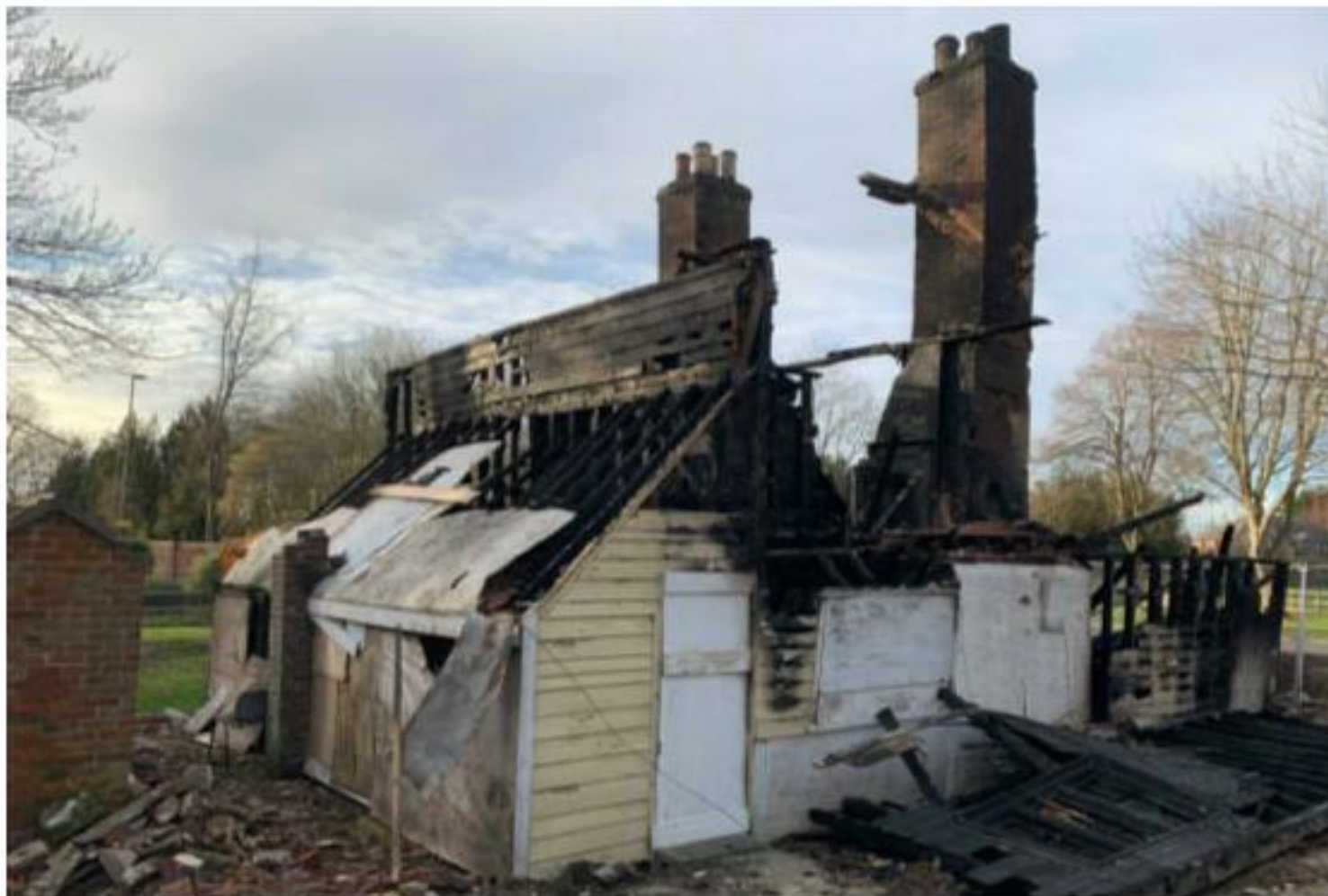
Figure 3: Post-Fire Damage (Jan 2019)
