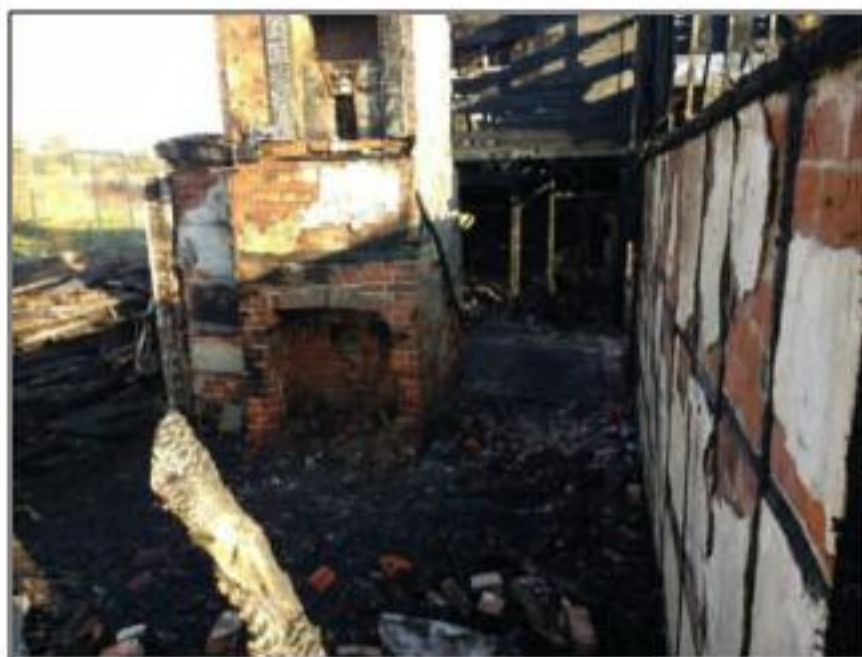
Figure 24: The cottages after the devastating fire (Jan, 2019)
