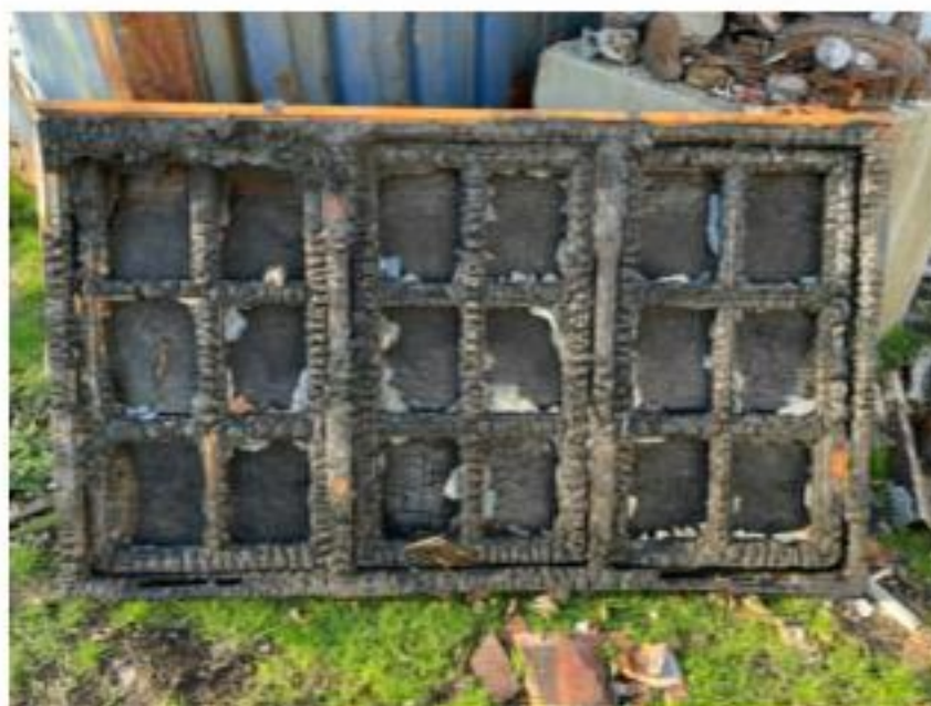
Figure 1: Window destroyed by the fire at 59 and 61 Langstone Road (Jan 2019)
