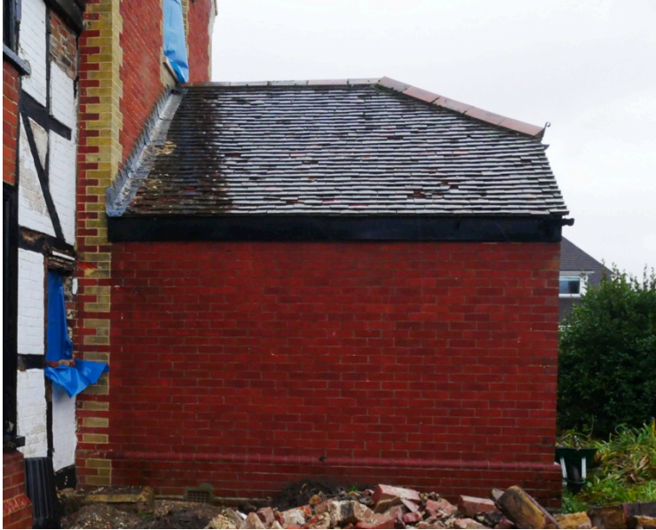
Extension to rear – southern roof slope with broken , missing and delaminated tiles.
