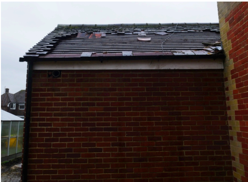
Extension to rear – southern roof slope with broken , missing and delaminated tiles. Exposed NW side with partially stripped roof slope.
