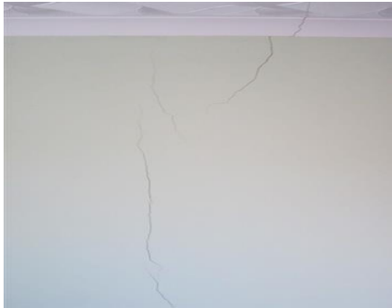
Lounge - Main crack damage to right hand elevation - junction of extension and main building
