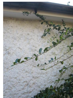
Left hand elevation main house - tapering diagonal crack damage
