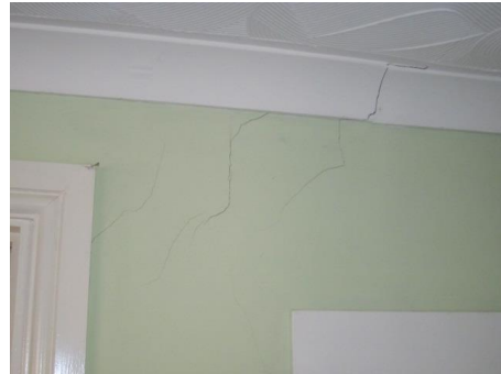
Lounge - Crack damage - towards the front elevation of the extension at the junction of the main building
