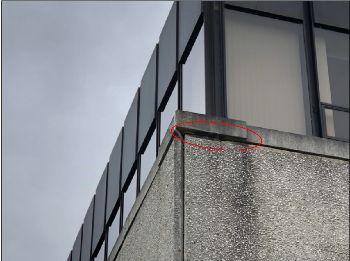
Figure 14. A gap at the south eastern corner of Building 1.
