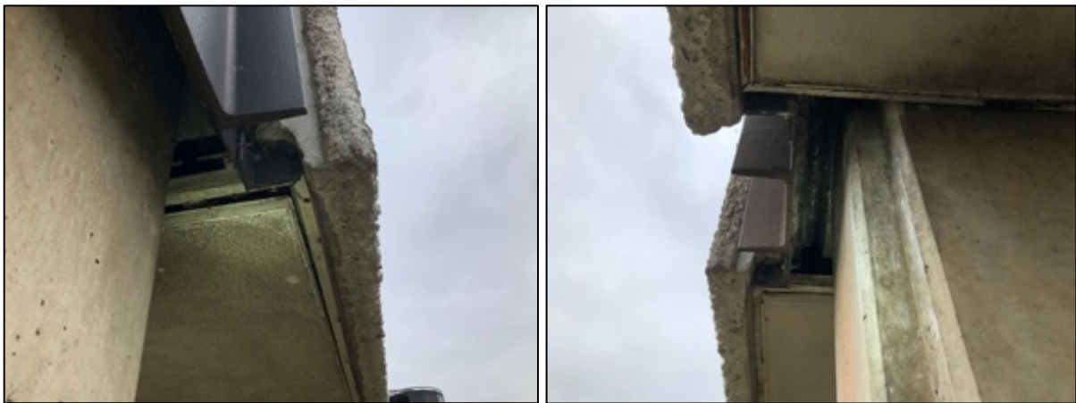
Figure 17. Further crevices visible around the concrete pillars supporting Building 2.
