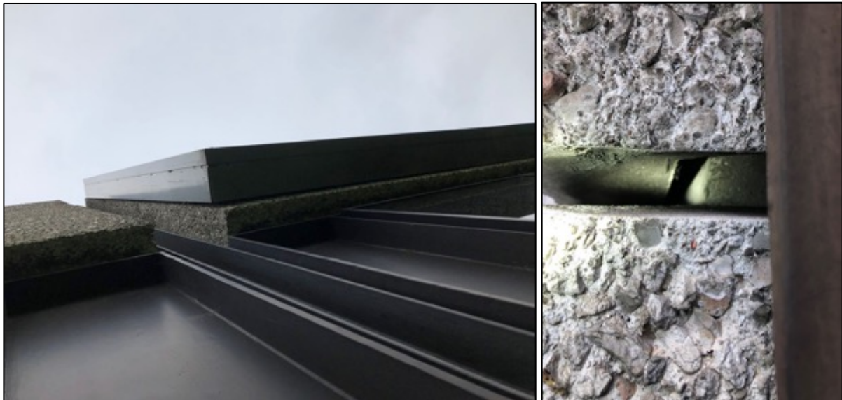
Figure 19. Left - A crevice behind a metal sign on the northern face of Building 3. Right – The gap present between the concrete cladding panels.
