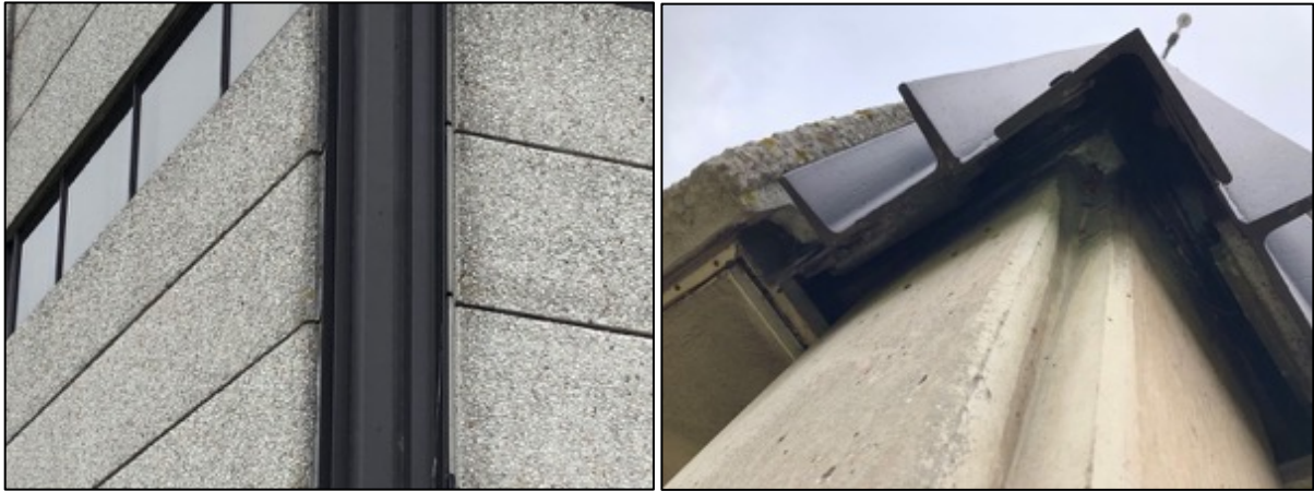
Figure 16. Left – crevices visible in-between cladding panels on Building 2 Right – gaps visible around concrete support pillars at Building 2.
