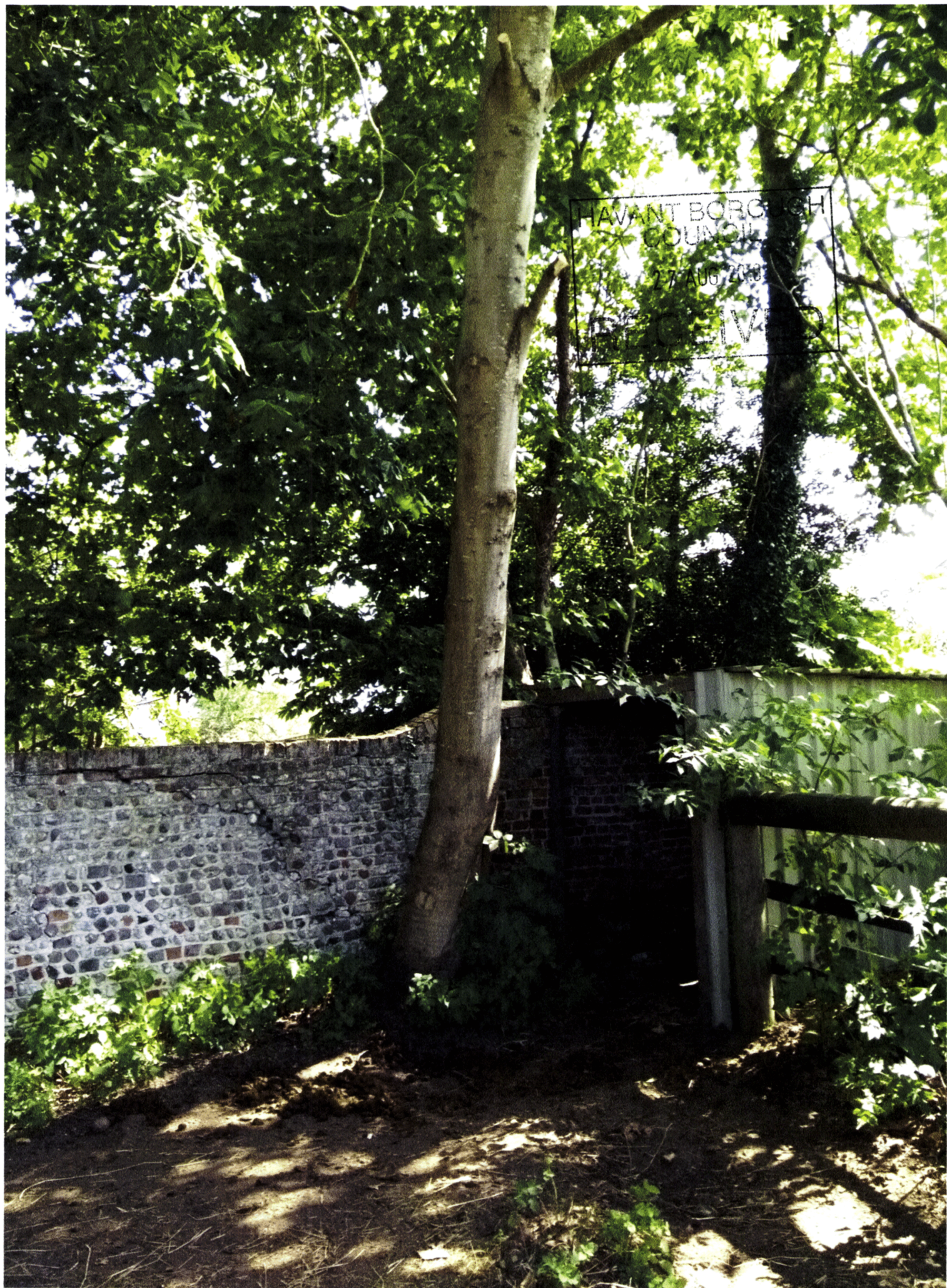
ROOT GROWING UNDER WALL CRACKING AND DAMAGING WALL
