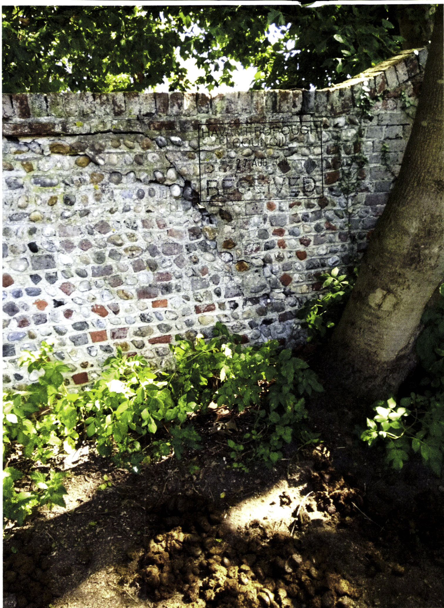
THE OLD RECTORY. ROOT IS GOING UNDER CRACKING WALL
