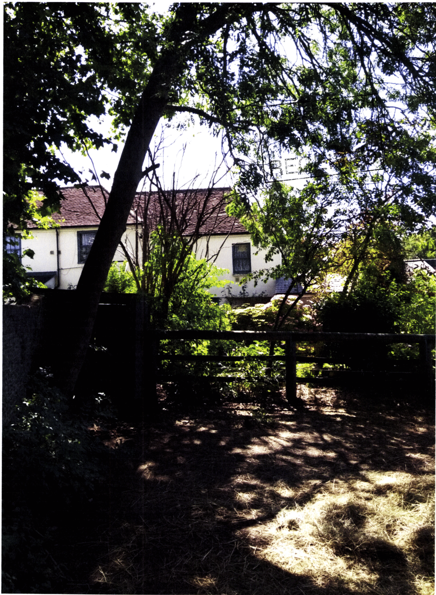
TREE LEANING TOWARDS RECTORY ANNEX ROOT GOING UNDER WALL
