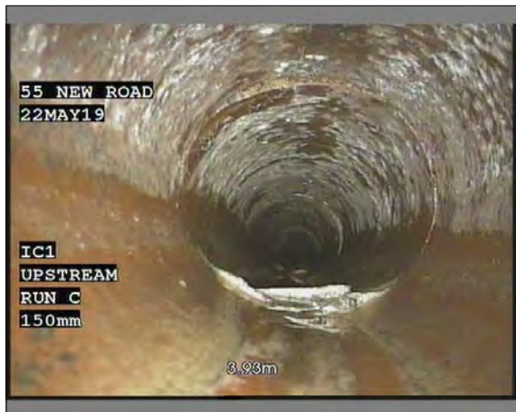
Photo: 003.JPG, VCR No.: 00003 3.93m, Scale, light at joint, from 5 to 7 o'clock
