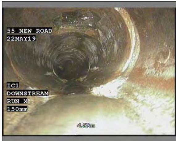
Photo: 006.JPG, VCR No.: 00004 4.59m, Broken sewer, from 11 to 2 o'clock
