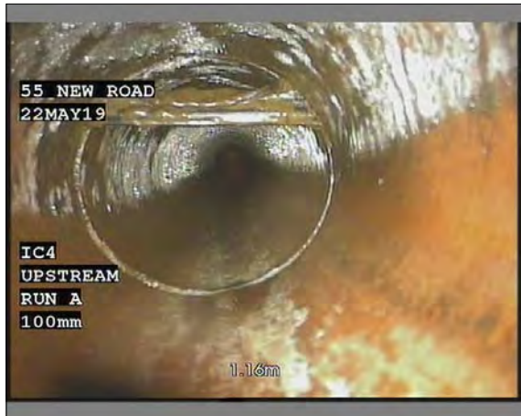
Photo: 009.JPG, VCR No.: 00006 1.16m, Obstruction, from 10 to 2 o'clock, 10% height loss
