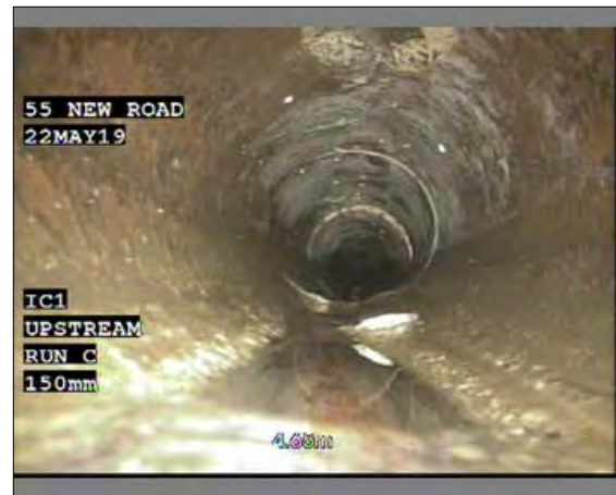
Photo: 004.jpg, VCR No.: 00003 4.65m, Hole in sewer, from 12 to 1 o'clock
