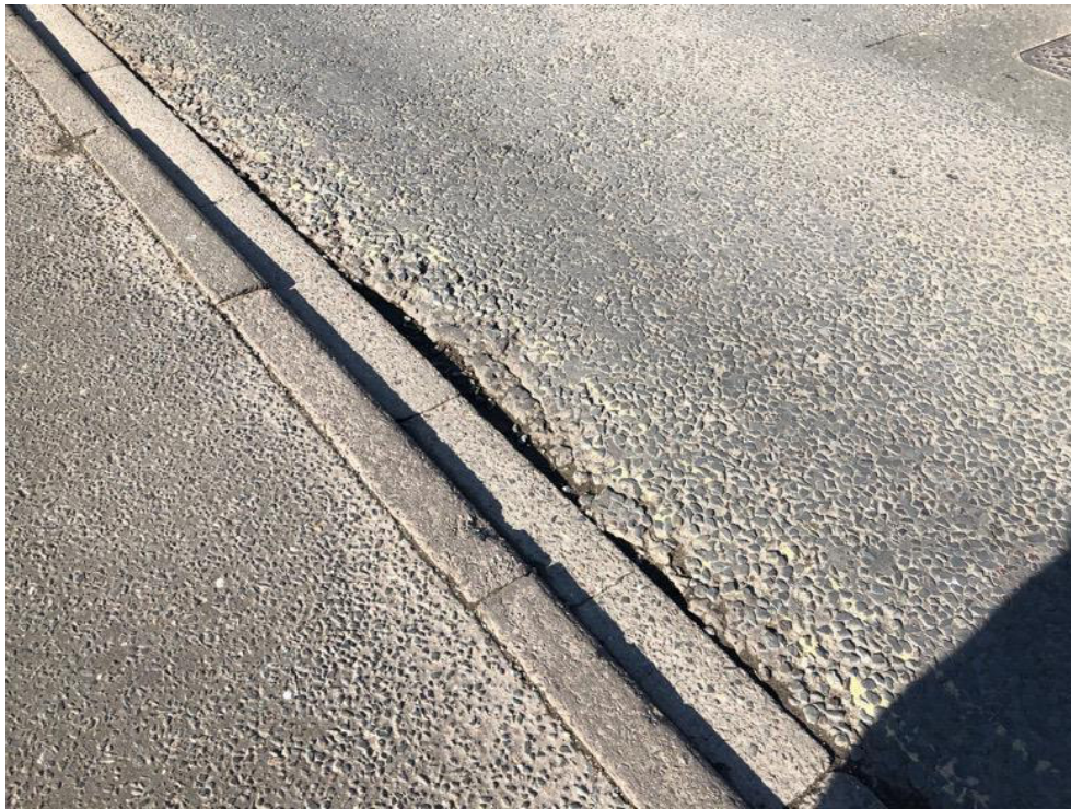
Photo 2: Edge of carriageway deteriorating adjacent to the proposed eastern access
