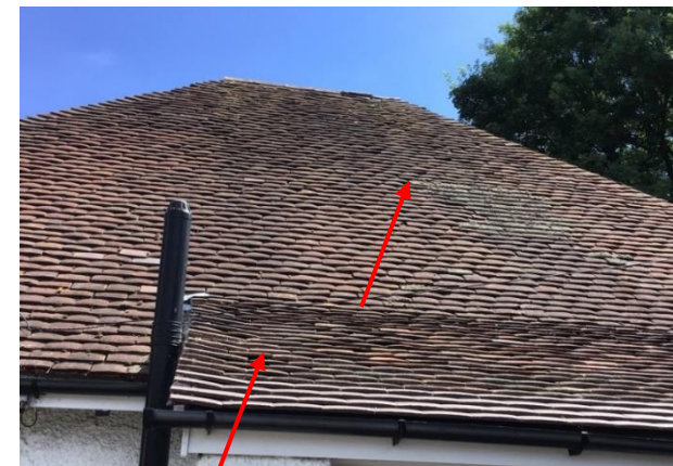
Plate 4.6: Gaps under roof tiles
