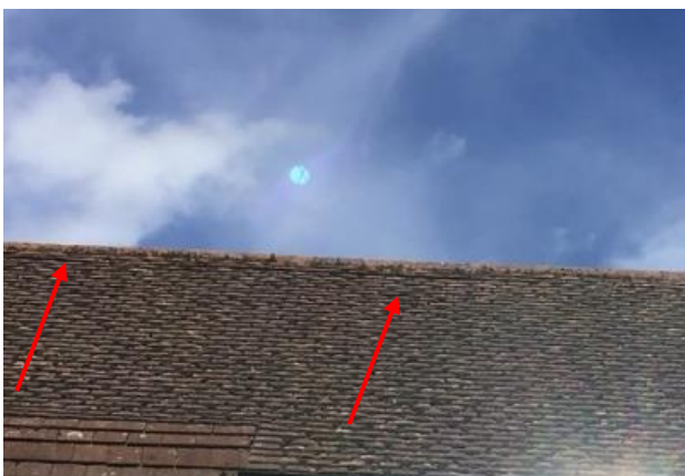
Plate 4.5: Gaps under roof tiles
