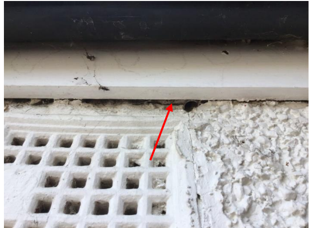
Plate 4.14: Gap between the wall and wooden fascia
