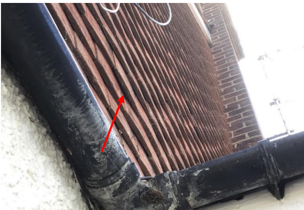
Plate 4.3: Gaps under hanging tiles
