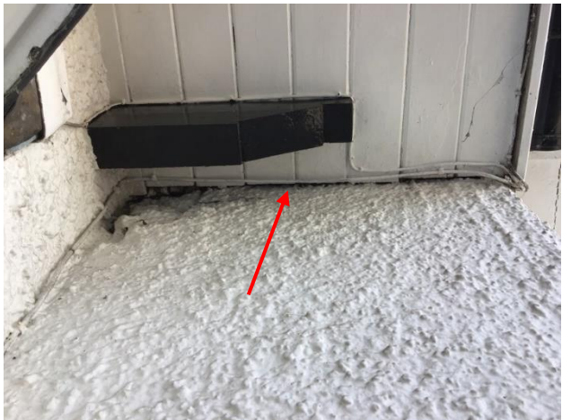
Plate 4.9: Gap between wall and soffit box
