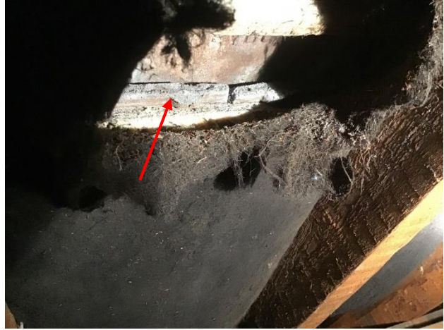
Plate 4.23: Damaged breathable membrane
