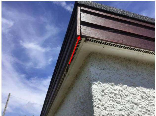
Plate 4.10: Gap at the soffit box
