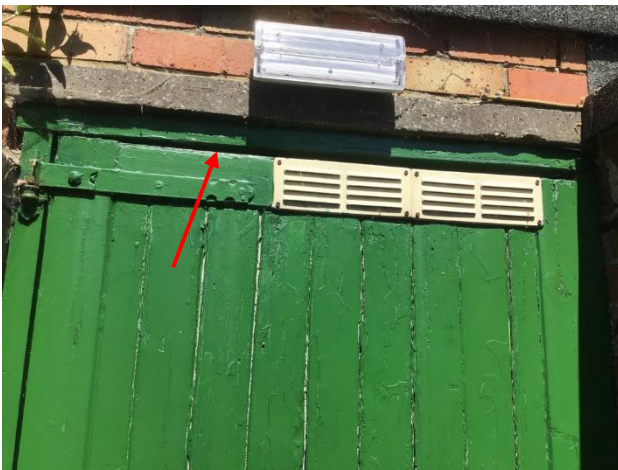
Plate 4.27: Gaps around the doorway
