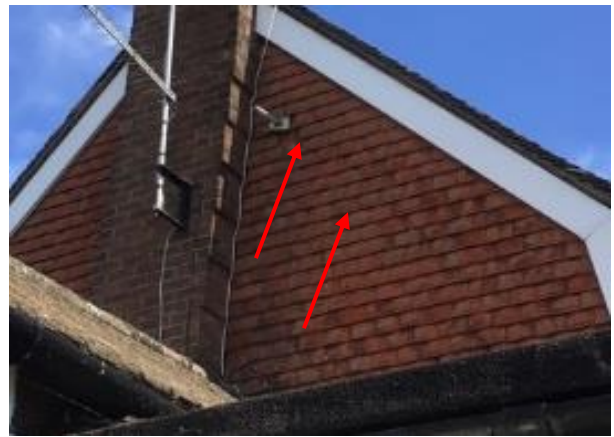
Plate 4.4: Gaps under hanging tiles
