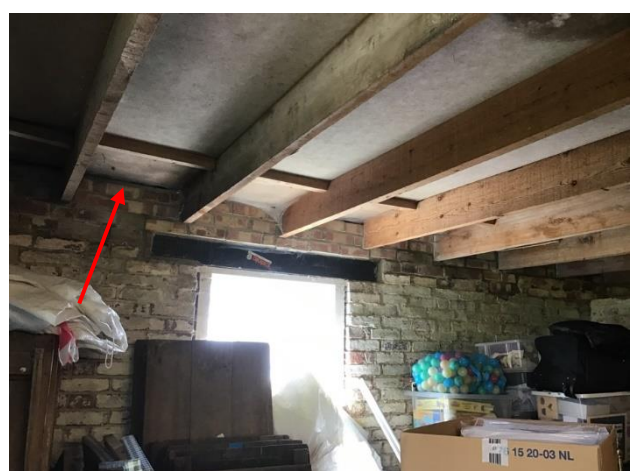
Plate 4.30: Gap between the ceiling and the wall
