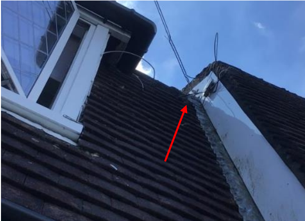
Plate 4.7: Lifted lead flashing
