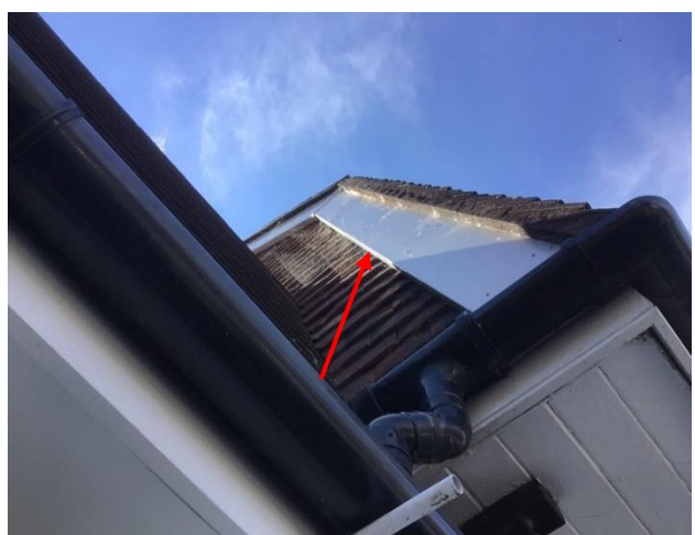
Plate 4.12: Gap between plastic fascia and hanging tiles
