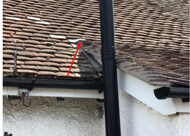
Plate 4.8: Lifted lead flashing
