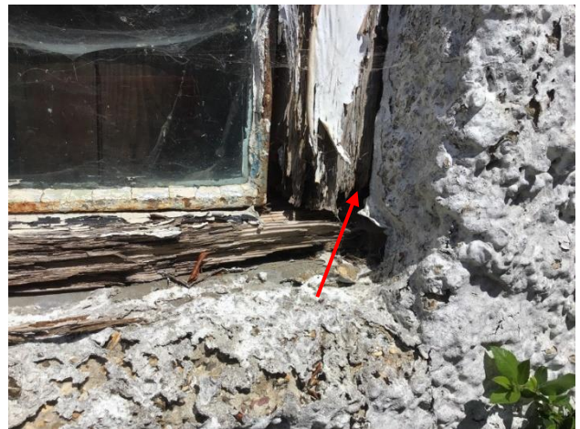
Plate 4.28: Gaps around the window frame
