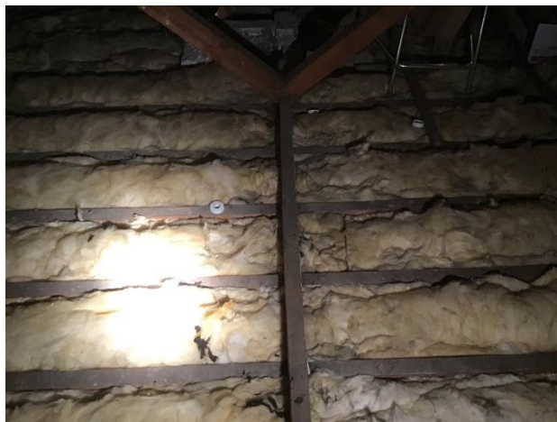
Plate 4.20: Fibre glass insulation
