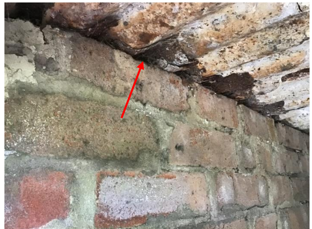
Plate 4.26: Gap between wall and the ceiling
