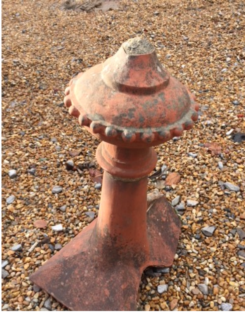
Damaged Terracotta finial to be replaced to match.
