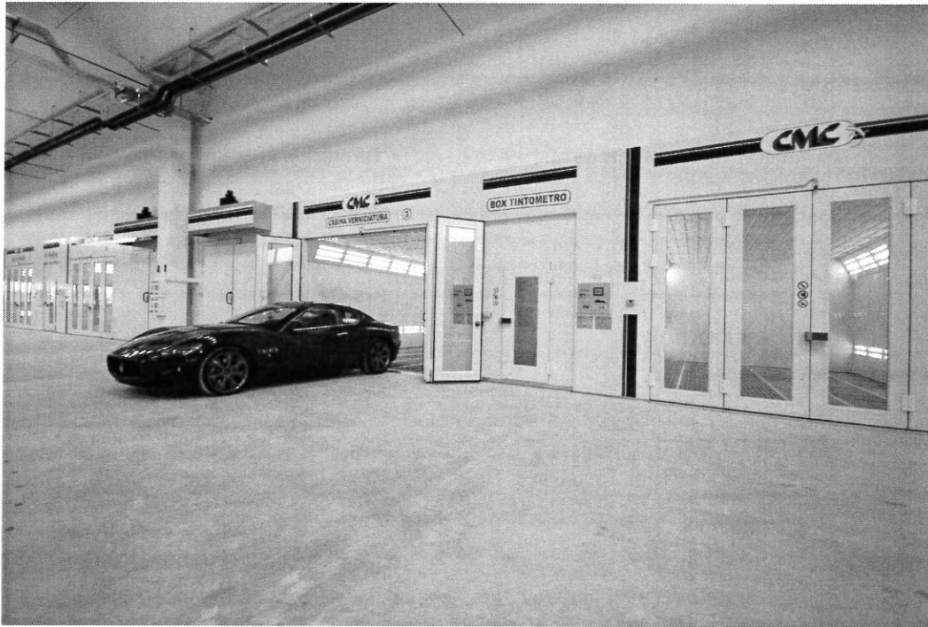
CMC spray booth installed in Modena, Italy
