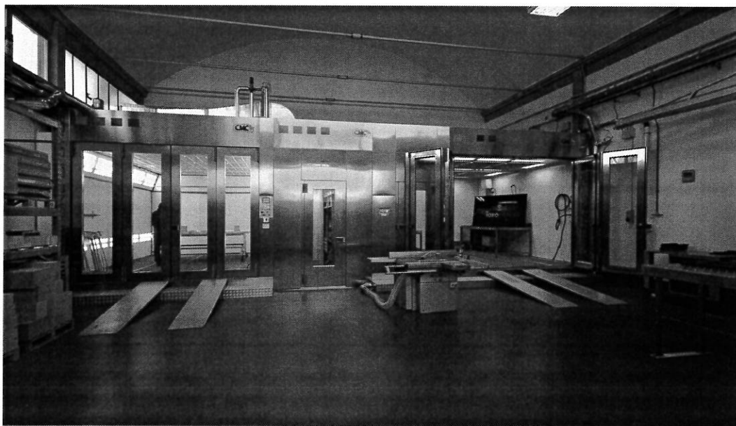
CMC spray booth and preparation equipment installed in the Scuderia Toro Rosso factory in Faenza, Italy
