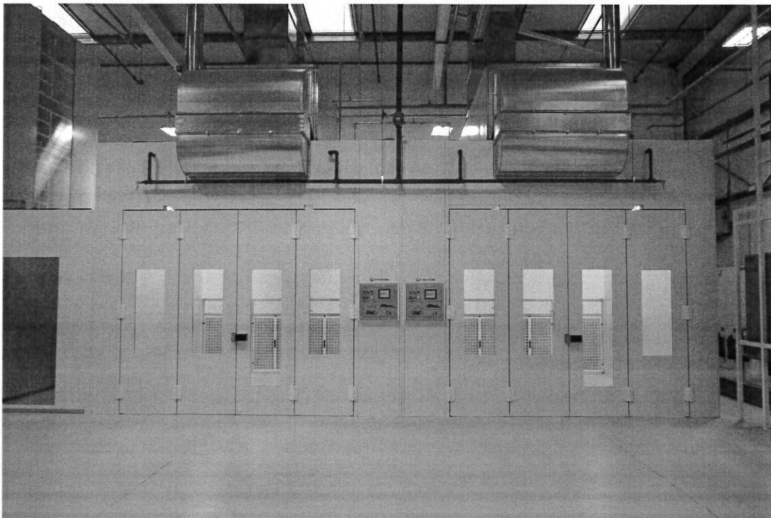
Twin 4m x 4m custom spray booth/ovens with roof mounted plant and touch screen control panels
