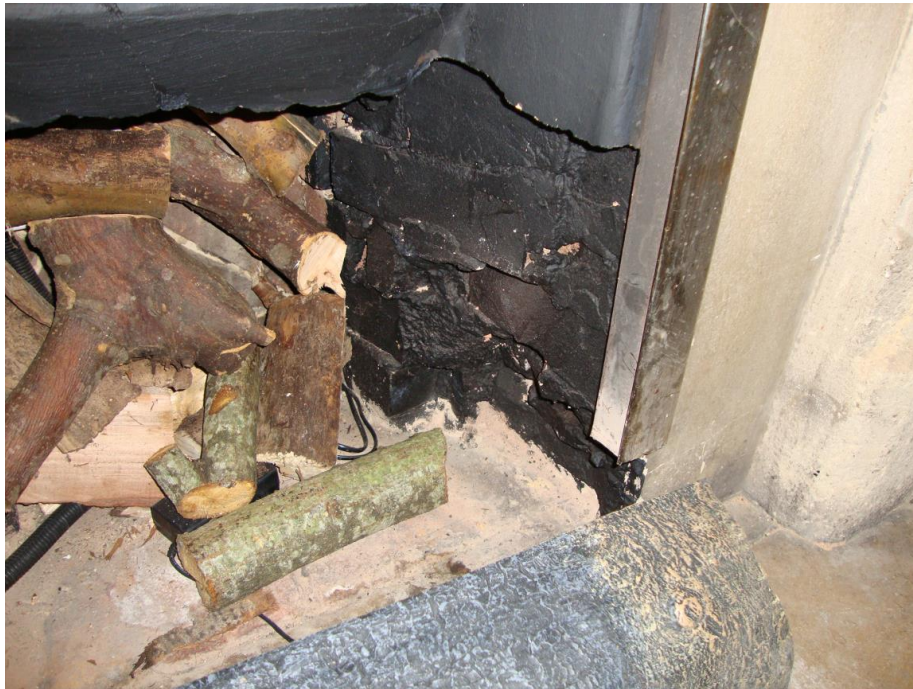
5.10 RHS of the fireplace showing modifications required in order to accommodate the gas fire.
