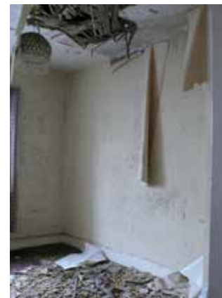
Room on eastern boundary - water damaged ceiling
