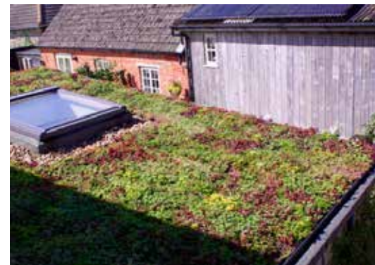
Sedum green roof, domestic http://www.sedumgreenroof.co.uk
