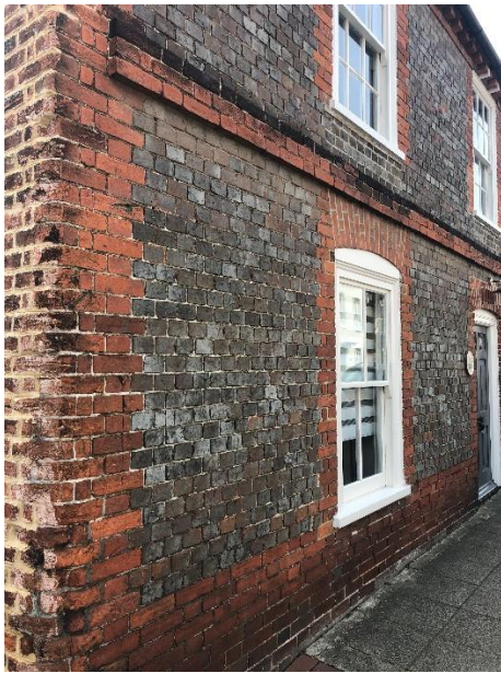
Figure 10: Property on King Street, Emsworth. displaying dark brickwork.
