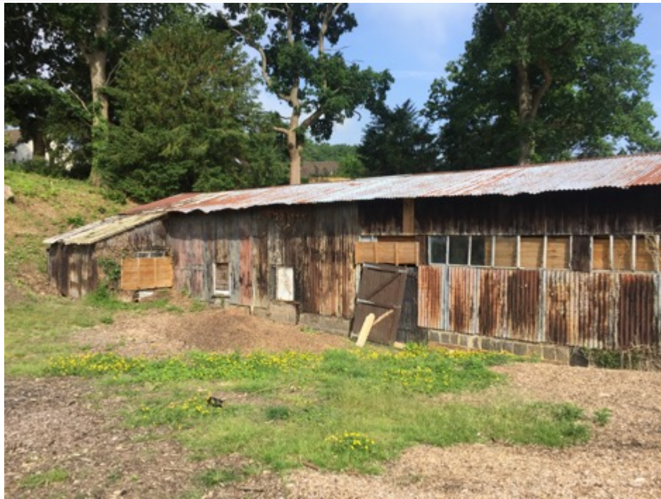
Photograph 3 Facing north, showing corrugated building in a poor state of repair located in the centre of the site.
