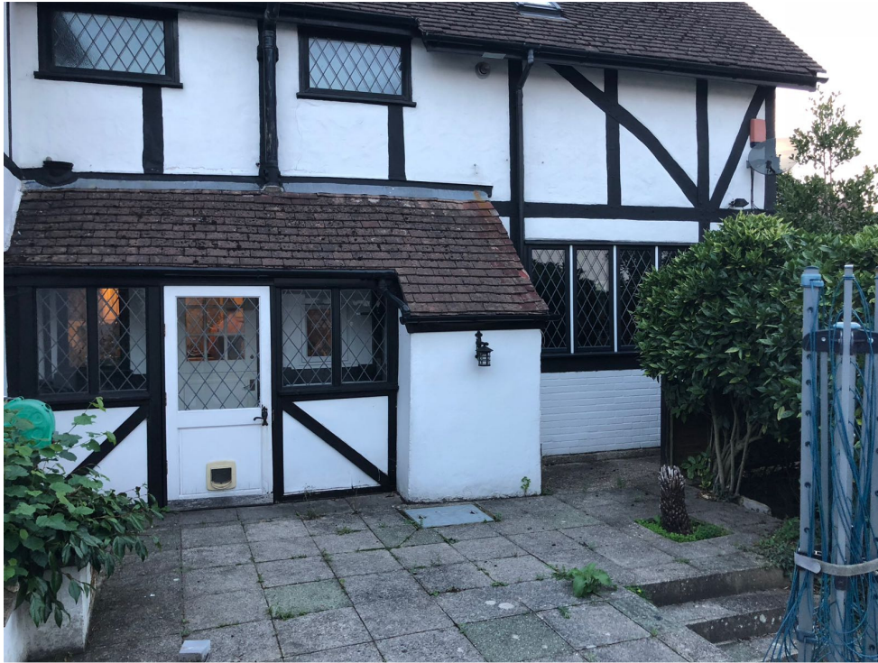
View of existing single storey poorly constructed extension/ lean too.
