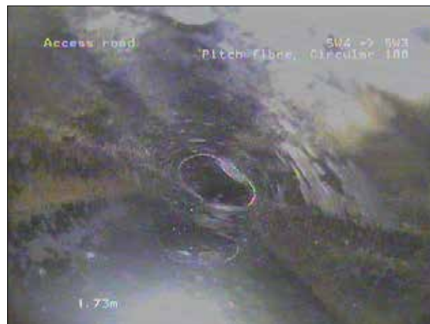
Photo: 190_3a, 00:00:00 1.73m, Deformed drain/sewer 30 %
