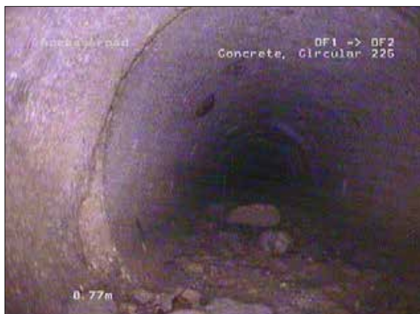
Photo: 119_3a, 00:00:00 0.77m, Settled deposits coarse 10 % cross-sectional area loss
