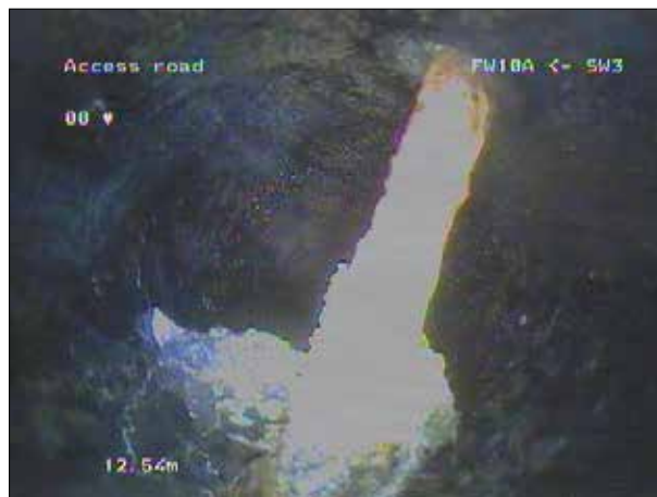
Photo: 176_7a, 00:00:00 12.54m, Survey abandoned, Remark: protruding metal in line
