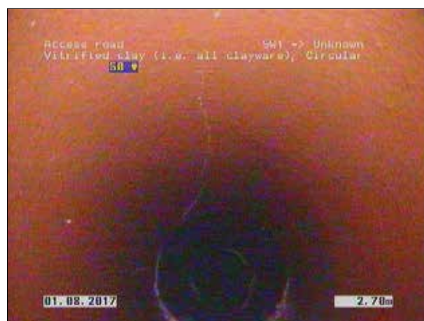
Photo: 81_8a 2.7m, Crack Longitudinal at 12 o'clock
