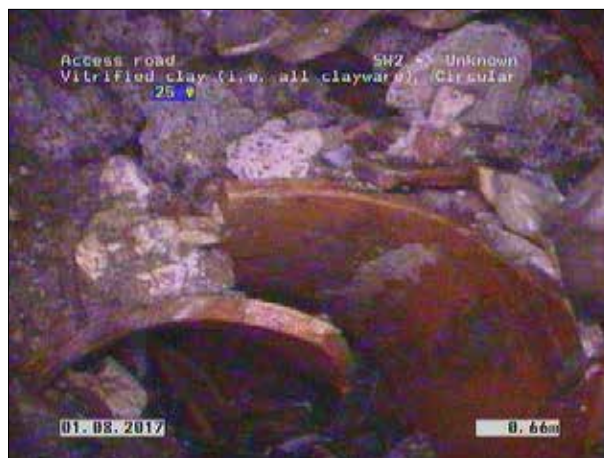
Photo: 99_5a 0.66m, Collapsed drain/sewer Remark: collapsed line
