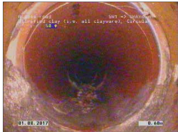
Photo: 66_3a 0.6m, Settled deposits fine 5 % cross-sectional area loss, Start
