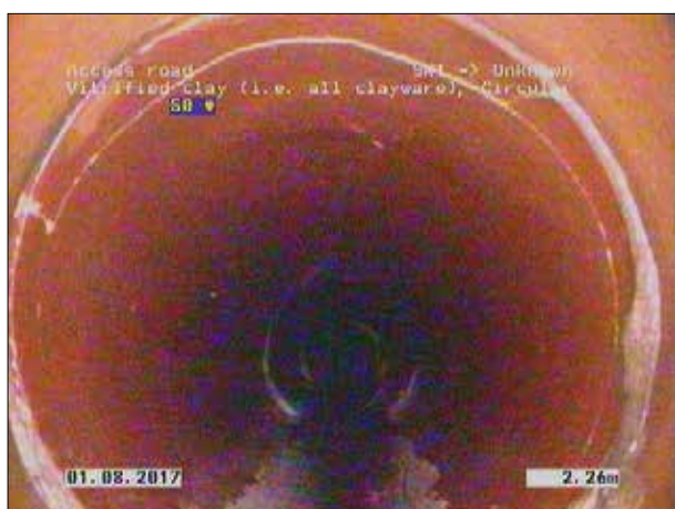
Photo: 80_7a 2.26m, Circumferential Fracture at joint from 09 to 05 o'clock
