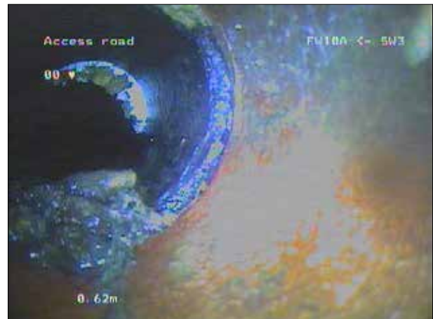
Photo: 172_3a, 00:00:00 0.59m, Material of drain/sewer changes to Pitch fibre
