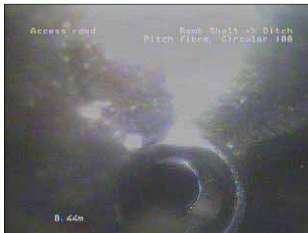
Photo: 216_7a, 00:00:00 8.44m, Survey abandoned, Remark: deformed PF
