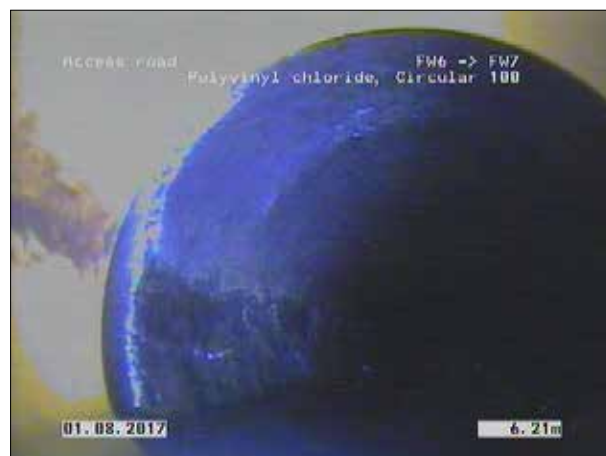
Photo: 7_3a 6.21m, Line of drain/sewer deviates right
