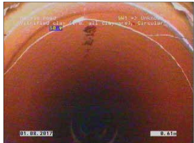
Photo: 76_3a 0.61m, Circumferential Fracture at joint from 07 to 03 o'clock
