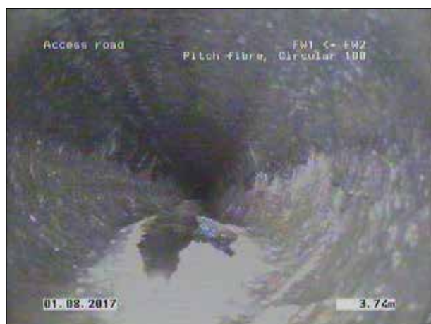
Photo: 1_4a 3.74m, Deformed drain/sewer 10 %
