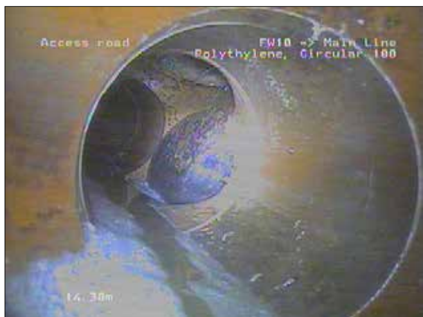
Photo: 154_8a, 00:00:00 14.38m, Line of drain/sewer deviates left
