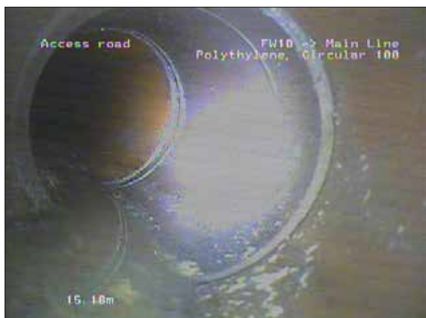
Photo: 156_10a, 00:00:00 15.18m, Line of drain/sewer deviates left
