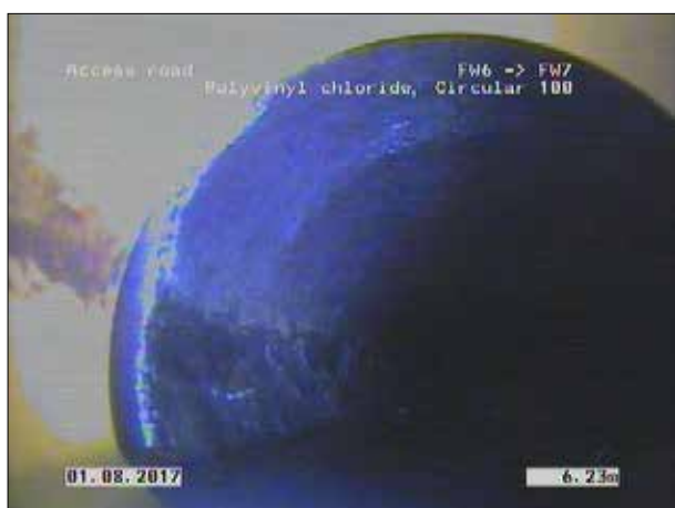
Photo: 7_4a 6.21m, Material of drain/sewer changes to Pitch fibre
