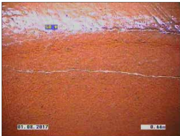
Photo: 76_3b 0.61m, Circumferential Fracture at joint from 07 to 03 o'clock
