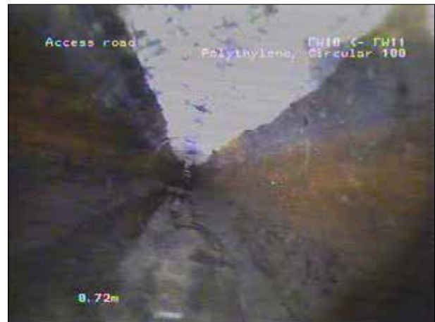
Photo: 24_3a, 00:00:00 0.72m, Attached deposits encrustation from 04 to 07 o'clock 5 % cross-sectional area loss, Start
