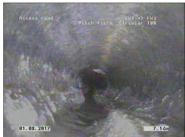
Photo: 15_5a 7.14m, Deformed drain/sewer 5 % Remark: blistered pitch fiber
