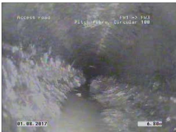
Photo: 14_4a 6.8m, Attached deposits encrustation from 04 to 08 o'clock 5 % cross-sectional area loss
