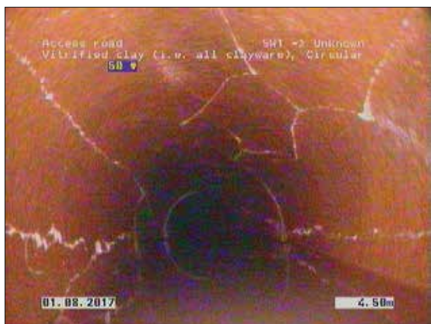
Photo: 90_17a 4.5m, Multiple Cracks from 09 to 03 o'clock
