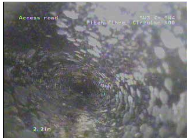
Photo: 186_3a, 00:00:00 2.21m, Deformed drain/sewer 20 %
