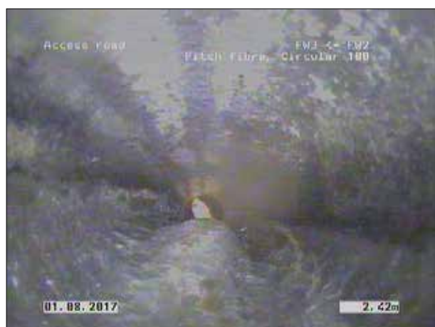
Photo: 104_4a 2.4m, Deformed drain/ sewer 30 % Remark: blistered PF
