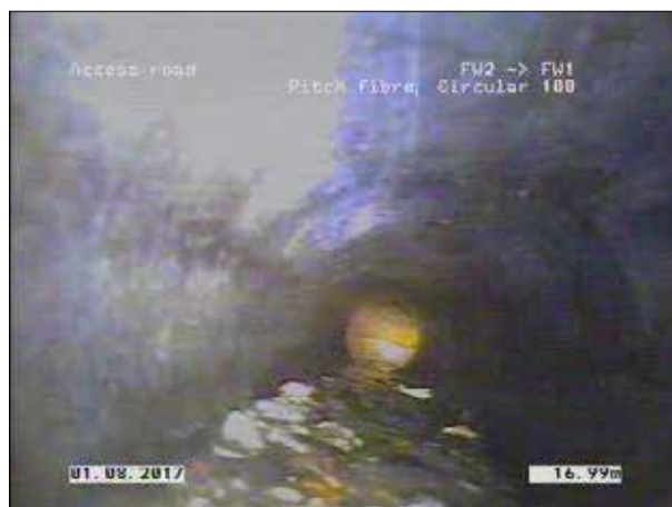
Photo: 35_15a 16.99m, Settled deposits coarse 5 % cross-sectional area loss
