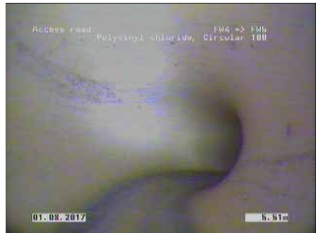
Photo: 111_3a 5.51m, Line of drain/sewer deviates right
