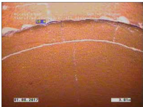
Photo: 83_10a 3.01m, Fracture longitudinal at joint at 12 o'clock
