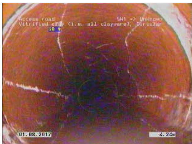
Photo: 88_15a 4.24m, Crack Longitudinal at joint at 02 o'clock
