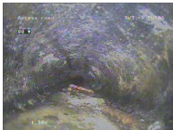
Photo: 179_3a, 00:00:00 1.3m, Material of drain/sewer changes to Pitch fibre
