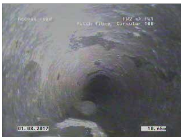
Photo: 3_8a 10.65m, Deformed drain/sewer 10 %
