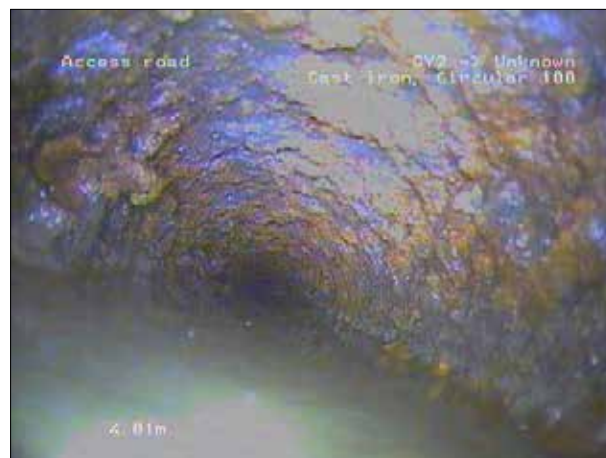
Photo: 126_6a, 00:00:00 4.01m, Loss of vision, camera under water
