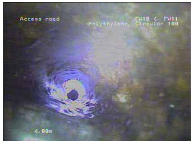
Photo: 168_6a, 00:00:00 3.98m, Attached deposits encrustation from 04 to 07 o'clock 10 % cross-sectional area loss, Start
