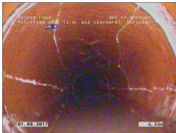
Photo: 87_14a 4.24m, Crack Longitudinal at joint at 11 o'clock
