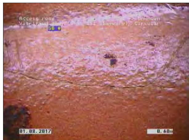
Photo: 67_4b 0.6m, Circumferential Fracture at joint from 07 to 03 o'clock
