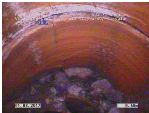
Photo: 97_3a 0.6m, Fracture longitudinal at joint at 11 o'clock
