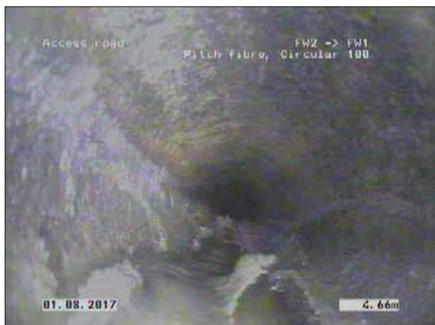
Photo: 3_4a 4.66m, Deformed drain/sewer 10 % Remark: blistered pitch fiber
