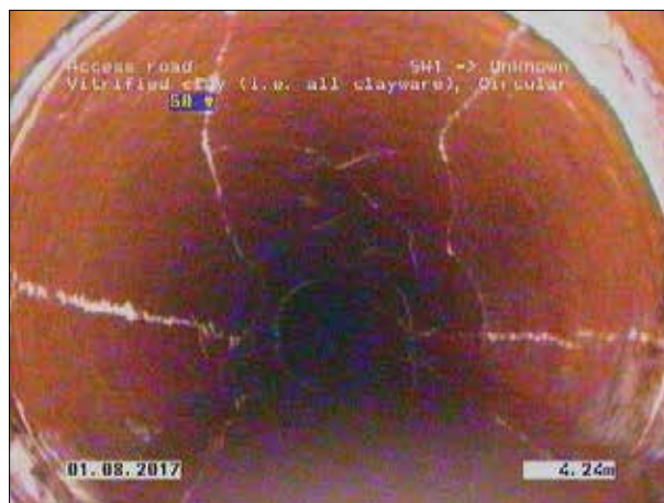
Photo: 89_16a 4.24m, Crack Longitudinal at joint at 04 o'clock
