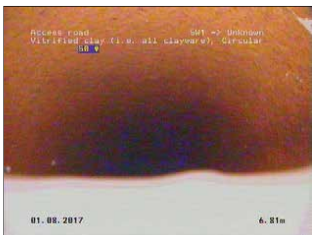
Photo: 94_21a 6.8m, Survey abandoned, Remark: water level to high and loss of traction
