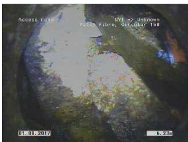
Photo: 73_4a 6.23m, Survey abandoned, Remark: collapsed line
