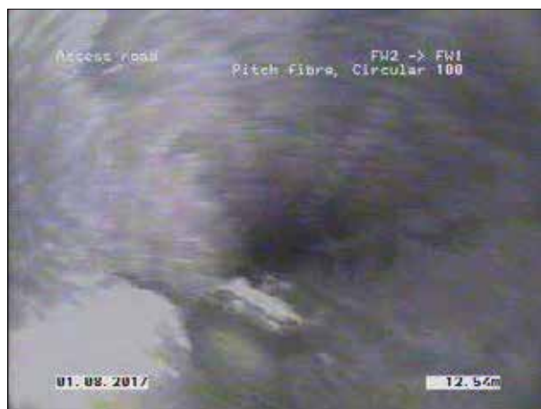
Photo: 31_11a 12.54m, Deformed drain/sewer 5 % Remark: blister pf
