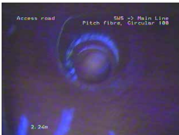
Photo: 30_4a, 00:00:00 2.24m, Line of drain/sewer deviates left
