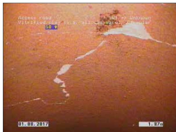
Photo: 79_6a 1.87m, Crack Circumferential at joint from 11 to 04 o'clock
