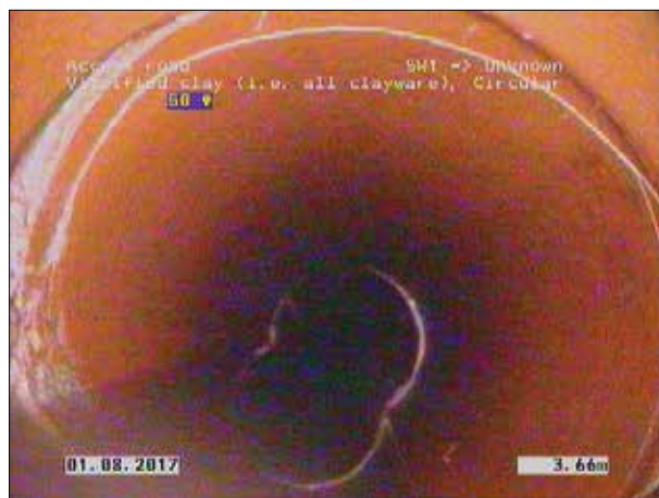
Photo: 84_11a 3.66m, Crack Circumferential at joint from 08 to 02 o'clock
