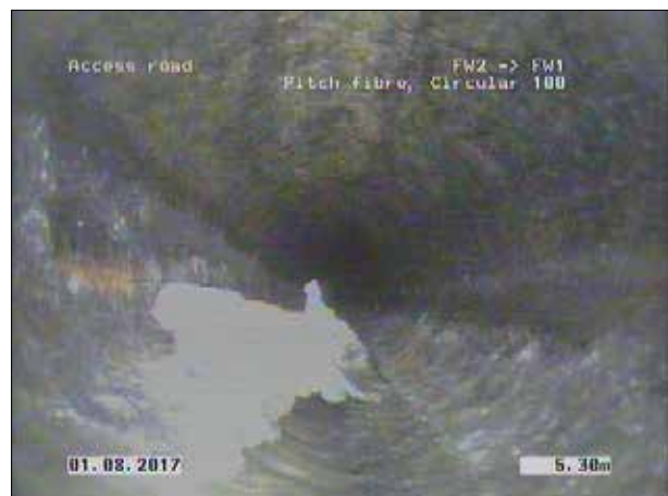
Photo: 3_5a 5.3m, Attached deposits encrustation from 04 to 07 o'clock 30 % cross-sectional area loss
