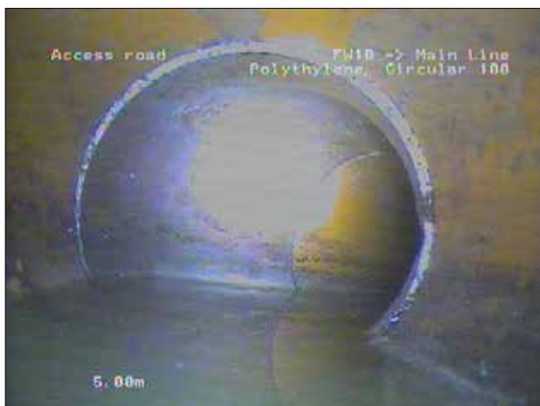
Photo: 150_4a, 00:00:00 5m, Line of drain/sewer deviates right
