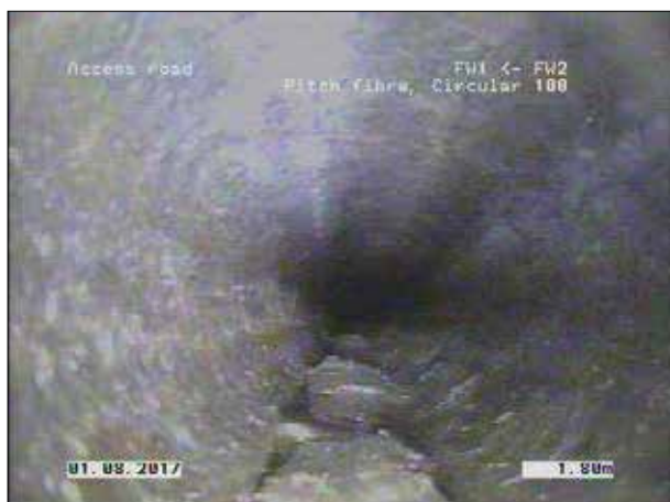
Photo: 1_6a 3.9m, Attached deposits encrustation at 06 o'clock 5 % cross-sectional area loss
