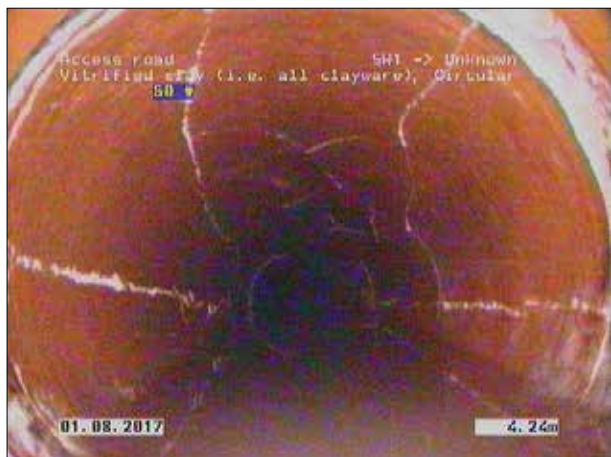
Photo: 86_13a 4.24m, Crack Longitudinal at 09 o'clock
