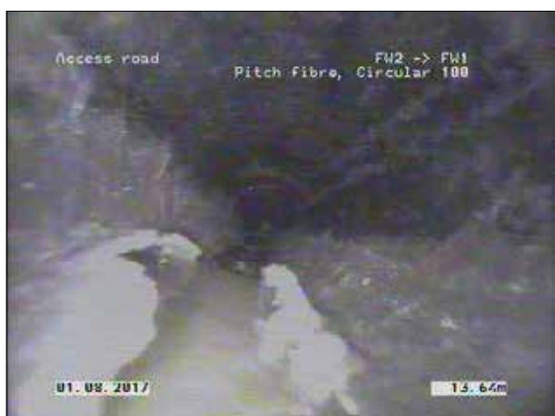
Photo: 32_12a 13.64m, Deformed drain/sewer 10 %
