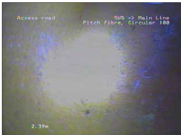
Photo: 30_6a, 00:00:00 2.39m, Line of drain/sewer deviates up
