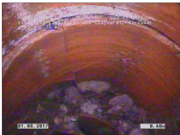
Photo: 98_4a 0.6m, Circumferential Fracture at joint from 11 to 02 o'clock
