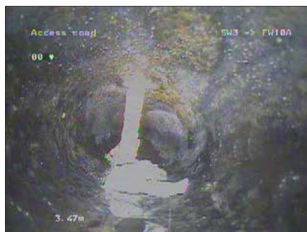
Photo: 183_5a, 00:00:00 3.47m, Survey abandoned, Remark: overlap to protruding metal in line
