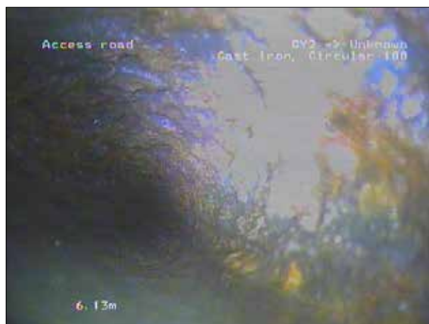
Photo: 128_8a, 00:00:00 6.13m, Survey abandoned, Remark: unable to push camera further
