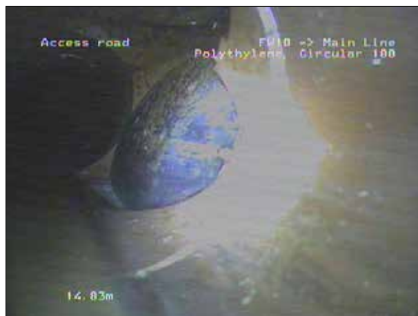
Photo: 155_9a, 00:00:00 14.83m, Connection at 12 o'clock, dia 100 mm
