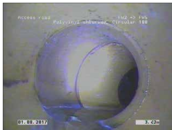
Photo: 4_3a 3.42m, Line of drain/sewer deviates right
