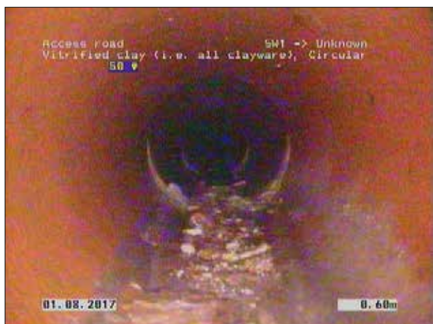
Photo: 68_5a 0.6m, Settled deposits coarse 5 % cross-sectional area loss
