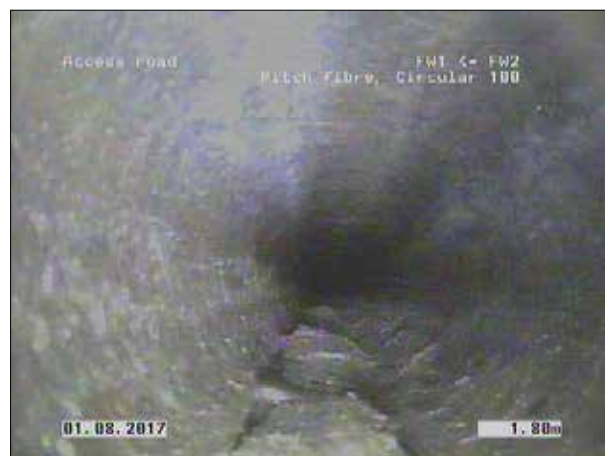
Photo: 3_3a 1.8m, Settled deposits hard or compacted 5 % cross-sectional area loss
