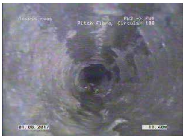
Photo: 30_10a 11.4m, Attached deposits encrustation from 02 to 11 o'clock 5 % cross-sectional area loss
