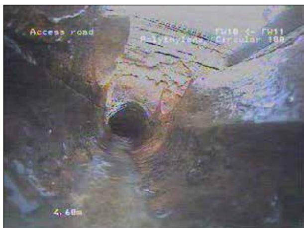
Photo: 169_7a, 00:00:00 4.59m, Attached deposits encrustation from 04 to 07 o'clock 10 % cross-sectional area loss Finish
