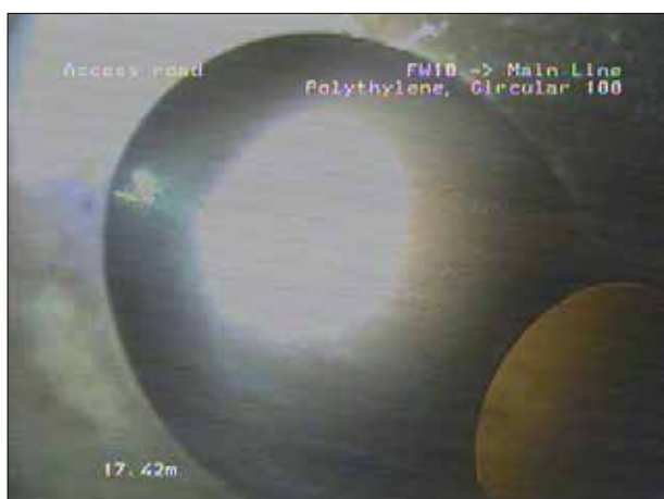
Photo: 158_12a, 00:00:00 17.42m, Major connection without manhole
