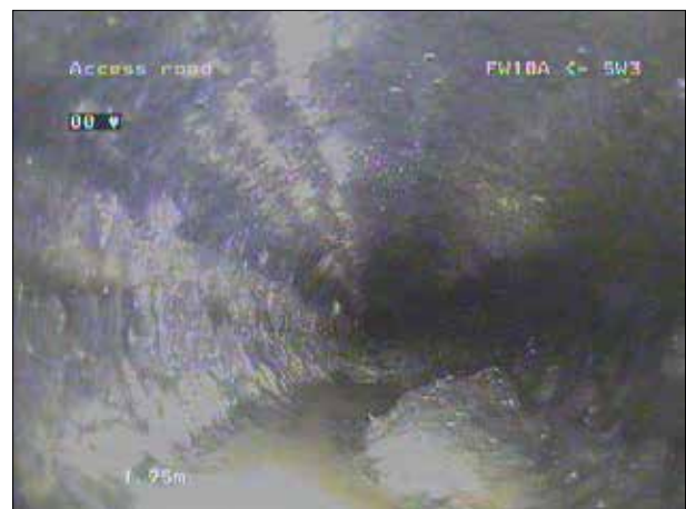
Photo: 174_5a, 00:00:00 1.95m, Deformed drain/sewer 10 % Remark: blistered pitch fiber
