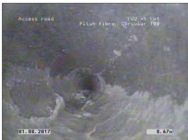
Photo: 3_6a 8.67m, Attached deposits encrustation from 03 to 09 o'clock 10 % cross-sectional area loss
