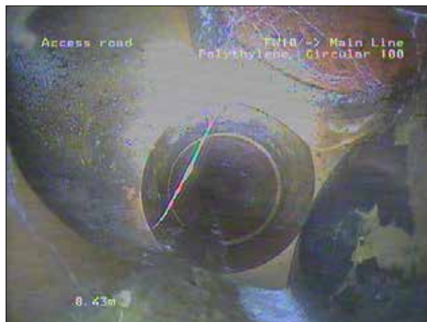
Photo: 153_7a, 00:00:00 8.43m, Connection at 12 o'clock, dia 100 mm
