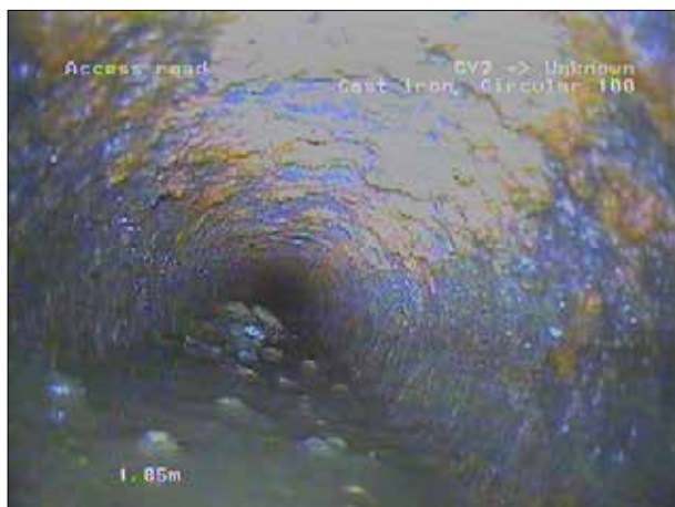
Photo: 124_4a, 00:00:00 1.85m, Settled deposits coarse 10 % cross-sectional area loss
