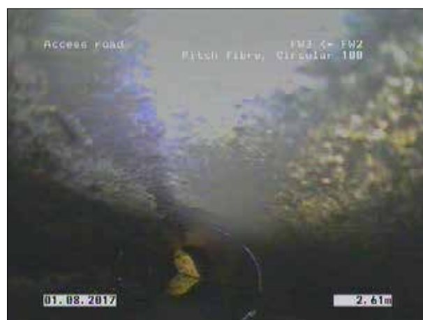
Photo: 105_5a 2.61m, Survey abandoned, Remark: deformed PF line
