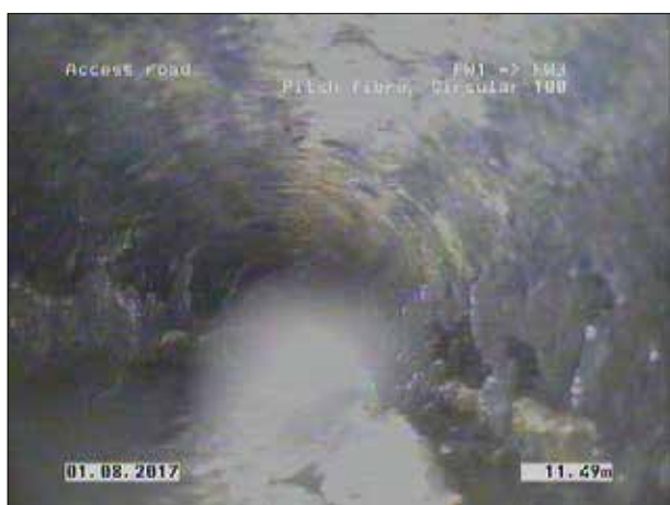
Photo: 18_8a 11.49m, Survey abandoned, Remark: due to 20%disformed blister PF
