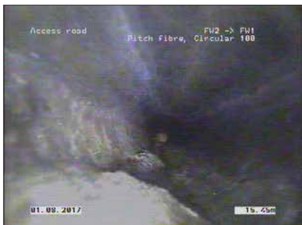
Photo: 34_14a 15.45m, Deformed drain/sewer 5 % Remark: blistered pf
