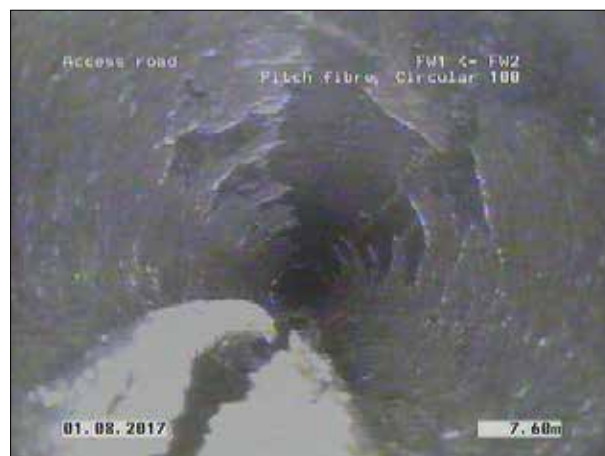
Photo: 1_7a 7.6m, Deformed drain/sewer 20 %
