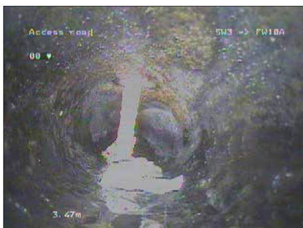
Photo: 182_4a, 00:00:00 3.47m, Other obstacles, other from, from 12 to 06 o'clock, 50 % cross-sectional area loss
