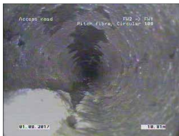
Photo: 3_9a 10.81m, Deformed drain/sewer 5 % Remark: blister pf
