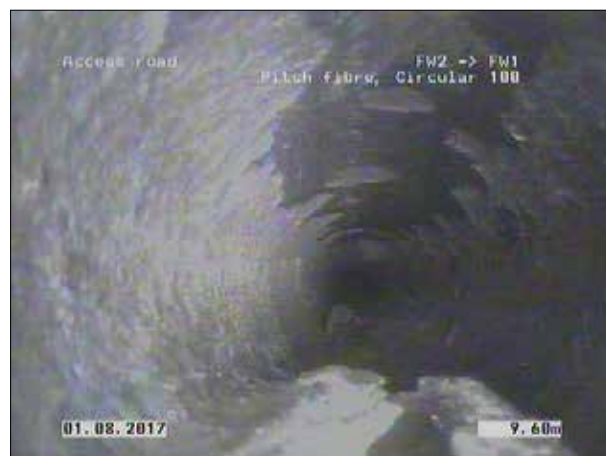
Photo: 3_7a 9.6m, Deformed drain/sewer 10 % Remark: blistered pitch fiber
