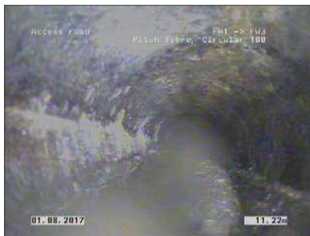
Photo: 17_7a 11.22m, Deformed drain/sewer 30 %
