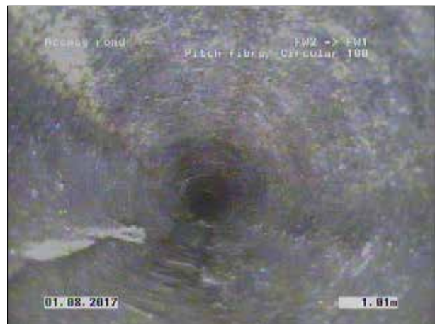
Photo: 3_3a 1.01m, Attached deposits encrustation at 07 o'clock 5 % cross-sectional area loss
