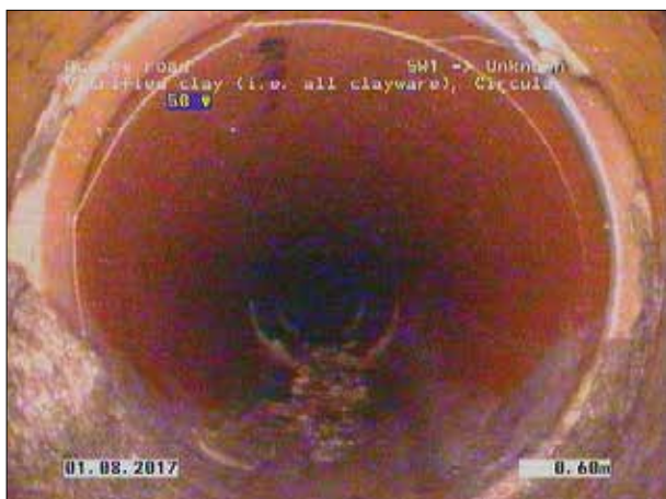
Photo: 67_4a 0.6m, Circumferential Fracture at joint from 07 to 03 o'clock
