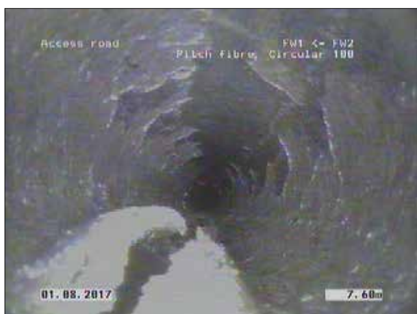
Photo: 1_8a 7.6m, Attached deposits encrustation from 05 to 07 o'clock 20 % cross-sectional area loss
