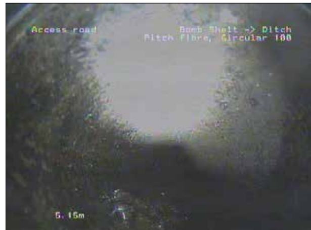
Photo: 31_3a, 00:00:00 0m, Line of drain/sewer deviates down
