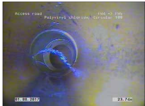
Photo: 17_5a 23.72m, Infiltration Running at 07 o'clock
