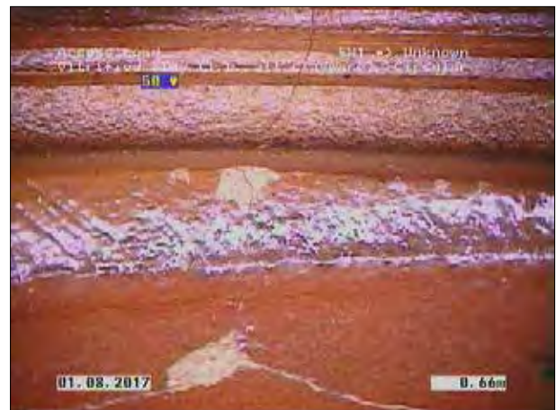
Photo: 77_4a 0.66m, Fracture longitudinal at joint at 12 o'clock
