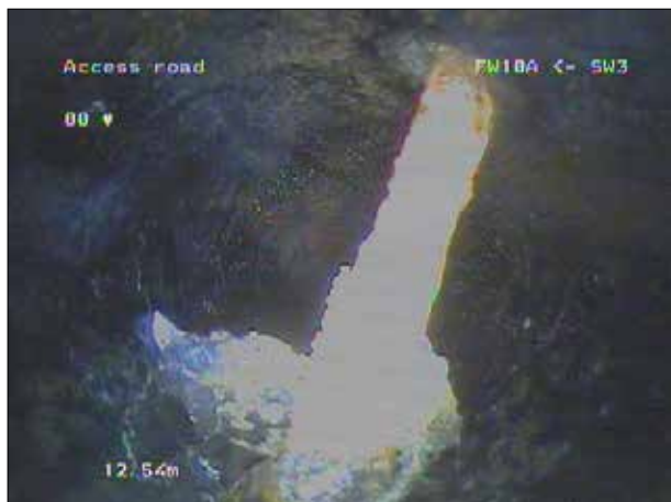
Photo: 175_6a, 00:00:00 12.54m, Other obstacles, other from, from 02 to 06 o'clock, 50 % cross-sectional area loss
