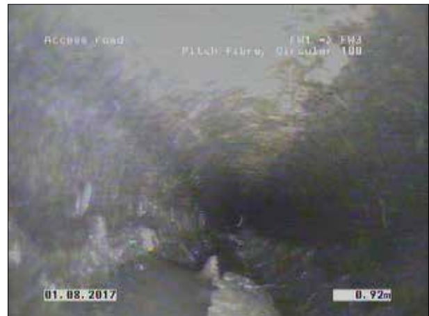
Photo: 13_3a 0.92m, Deformed drain/sewer 5 % Remark: blistered pitch fiber
