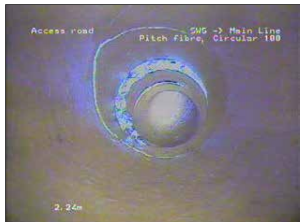
Photo: 30_5a, 00:00:00 2.24m, Crack Circumferential at joint from 04 to 02 o'clock
