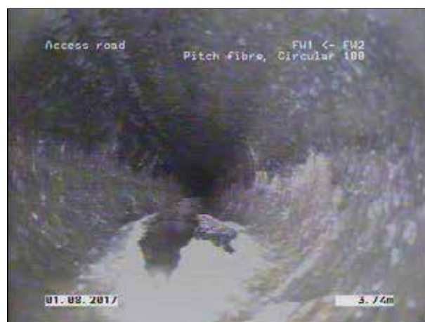
Photo: 10_5a 3.74m, Attached deposits encrustation from 05 to 07 o'clock 20 % cross-sectional area loss
