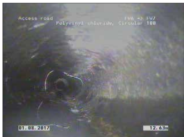
Photo: 7_6a 12.63m, Deformed drain/sewer 20 % Remark: unable to push past deformed line
