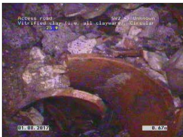
Photo: 100_6a 0.66m, Survey abandoned, Remark: collapsed line
