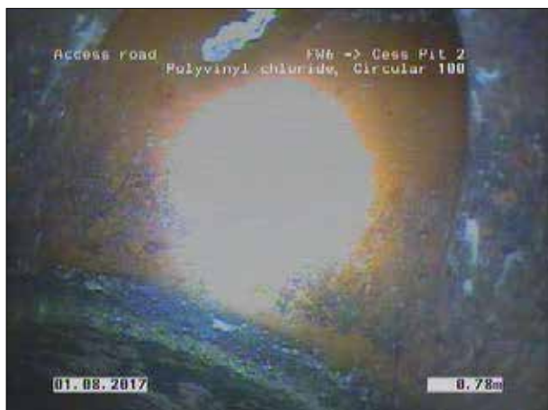
Photo: 47_3a 0.78m, Survey abandoned, Remark: back drop to cess pit
