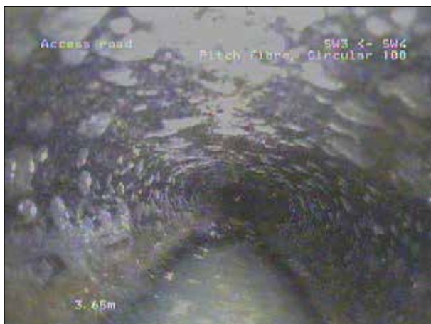
Photo: 187_4a, 00:00:00 3.65m, Survey abandoned, Remark: line to deformed to continue
