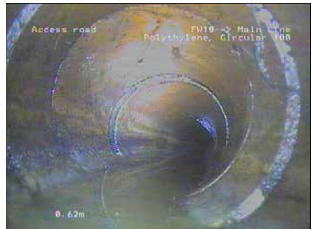
Photo: 149_3a, 00:00:00 0.58m, Line of drain/sewer deviates right
