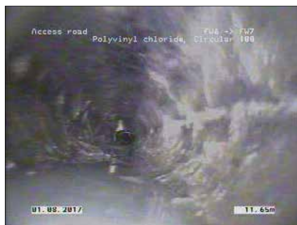
Photo: 7_5a 11.61m, Deformed drain/sewer 10 % Remark: blistered pf
