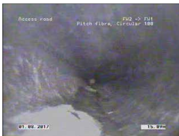
Photo: 33_13a 15.09m, Deformed drain/sewer 5 % Remark: blistered pf
