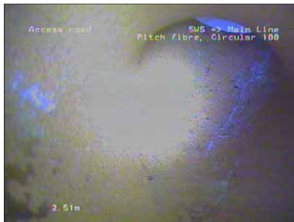
Photo: 30_7a, 00:00:00 2.51m, Survey abandoned, Remark: line goes up looks like a non return system
