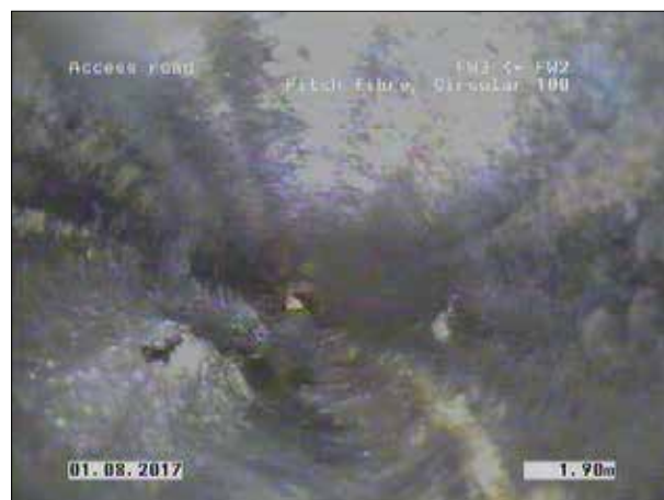
Photo: 103_3a 1.9m, Deformed drain/ sewer 10 % Remark: blistered PF
