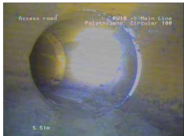
Photo: 151_5a, 00:00:00 5.51m, Line of drain/sewer deviates left
