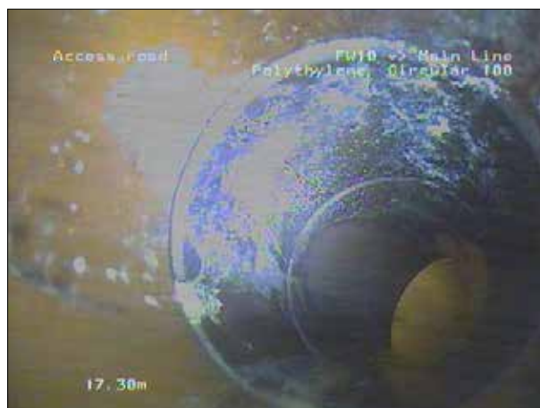
Photo: 157_11a, 00:00:00 17.3m, Line of drain/sewer deviates right
