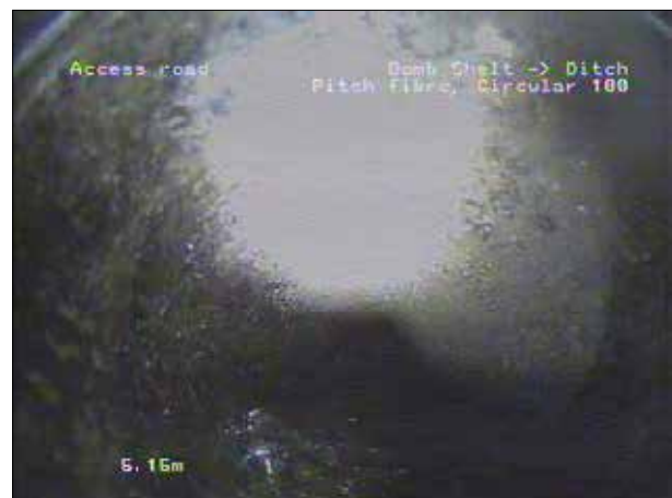
Photo: 209_5a, 00:00:00 5.15m, Settled deposits fine 10 % cross-sectional area loss, Start
