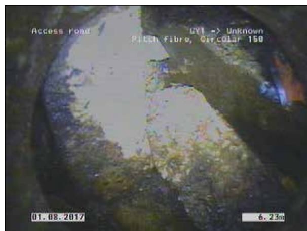
Photo: 72_3a 6.16m, Collapsed drain/sewer
