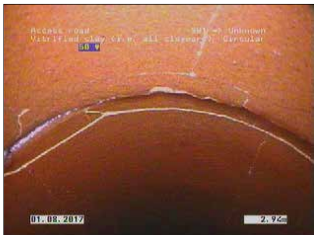
Photo: 82_9a 2.94m, Circumferential Fracture at joint from 09 to 03 o'clock
