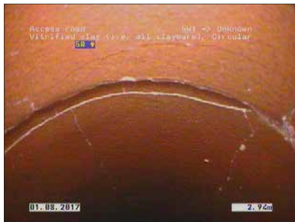
Photo: 82_9b 2.94m, Circumferential Fracture at joint from 09 to 03 o'clock
