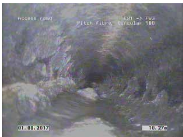
Photo: 16_6a 10.27m, Deformed drain/sewer 10 % Remark: blistered pitch fiber
