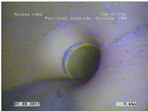
Photo: 17_4a 9.65m, Line of drain/sewer deviates right
