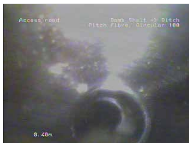
Photo: 214_5a, 00:00:00 8.4m, Deformed drain/sewer 20 % Remark: blistered PF
