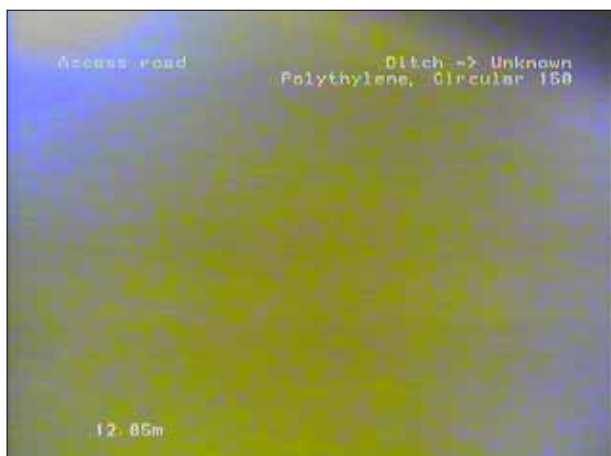
Photo: 228_7a, 00:00:00 12.85m, Loss of vision, camera under water
