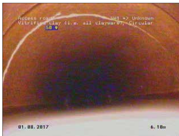
Photo: 92_19a 6.1m, Crack Circumferential at joint from 09 to 02 o'clock
