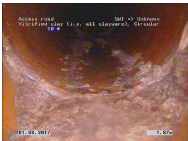
Photo: 78_5a 1.87m, Attached deposits encrustation from 04 to 07 o'clock 5 % cross-sectional area loss
