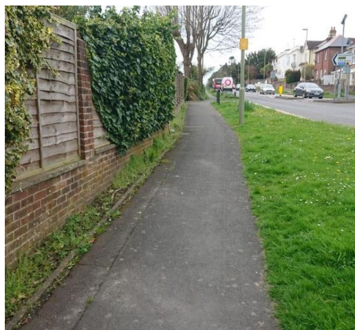
Photograph 49: Footway Conditions along Bedhampton Road
