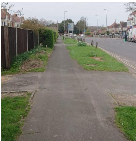
Photograph 48: Footway Conditions along Bedhampton Road
