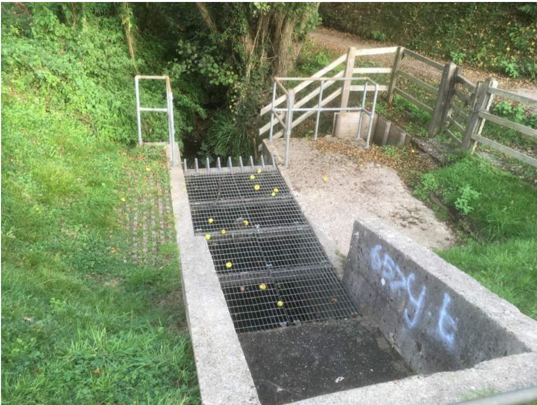
Plate 6. Drainage feature associated with stream adjacent south of the site (2018).
