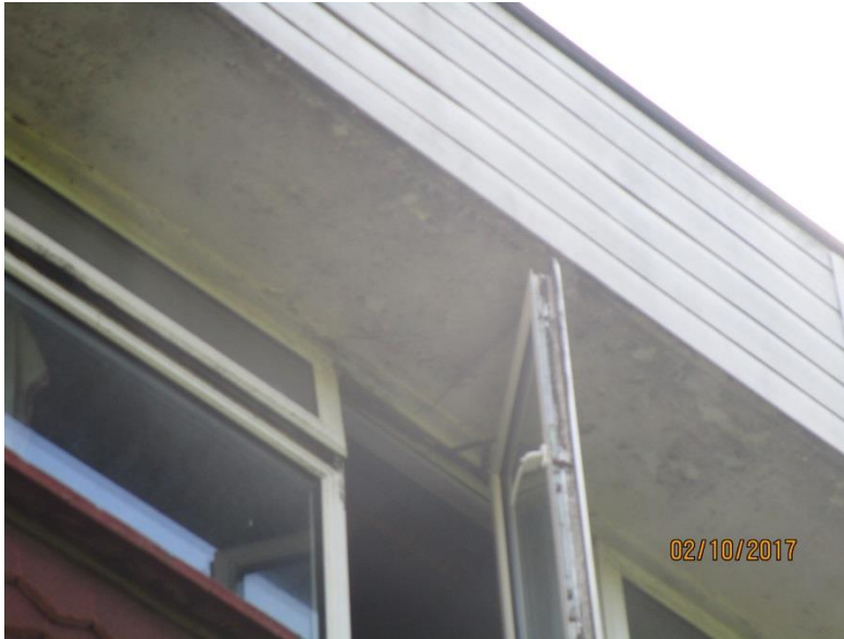
Photo 3 - Existing Facia Board and Soffit
