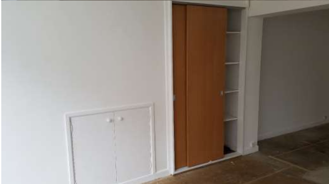
Adhoc and poorly constructed cupboards prior to light demolition.
