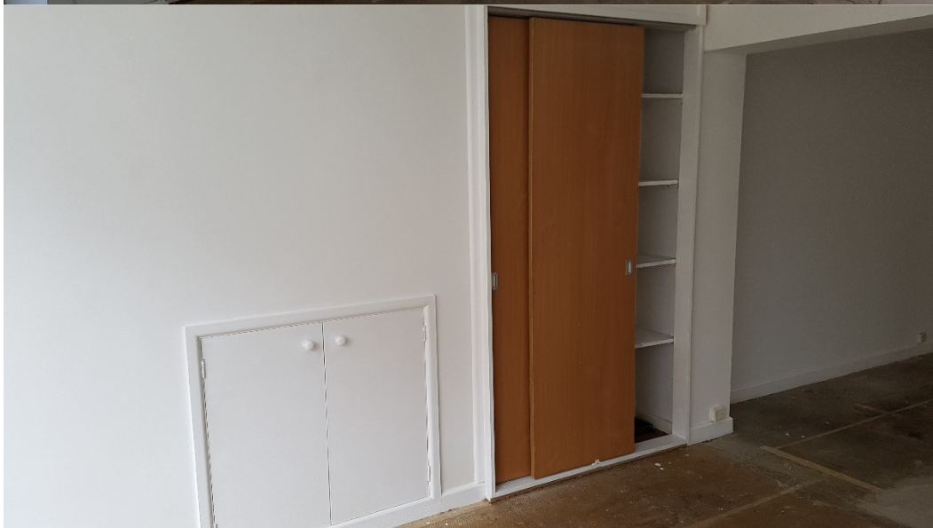
Adhoc and poorly constructed cupboards.
