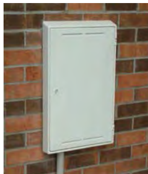
Cavity Meter Box
