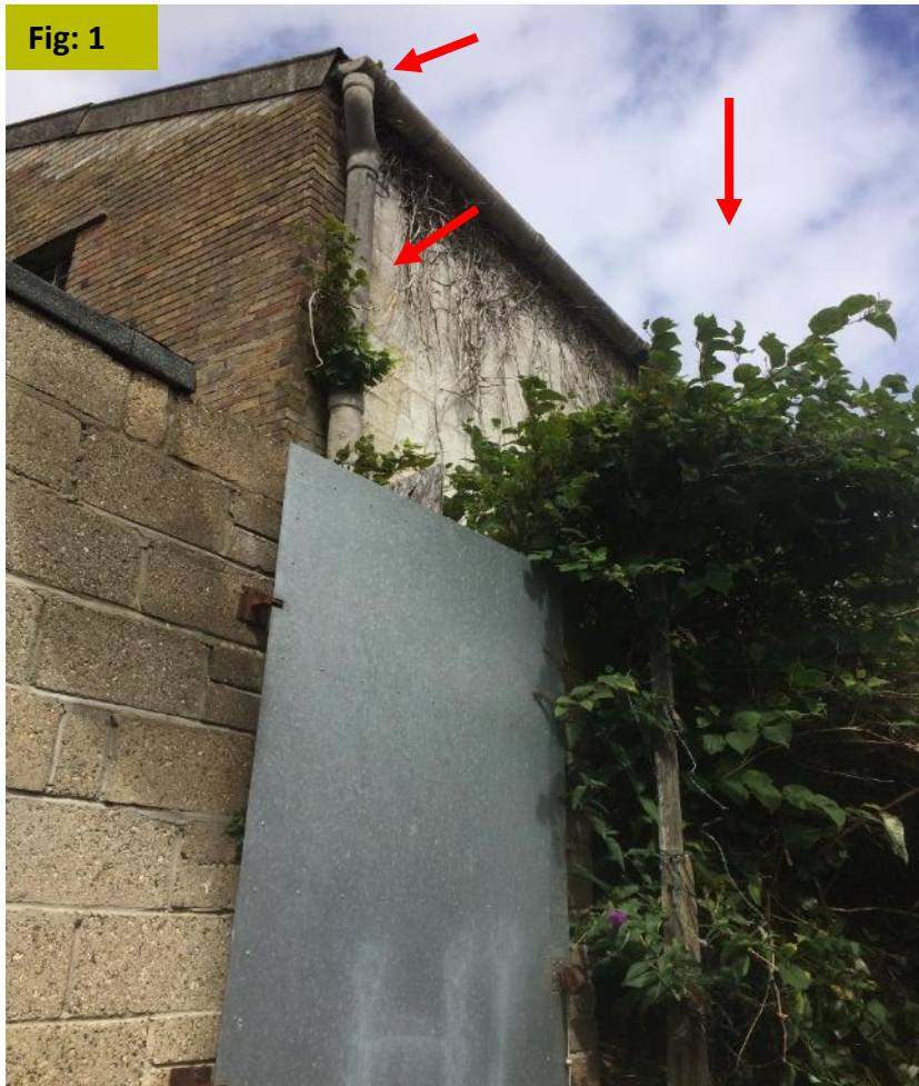
JK-2: Within boundary at: SU 6737 0792 – note the Japanese knotweed in the down pipe.
