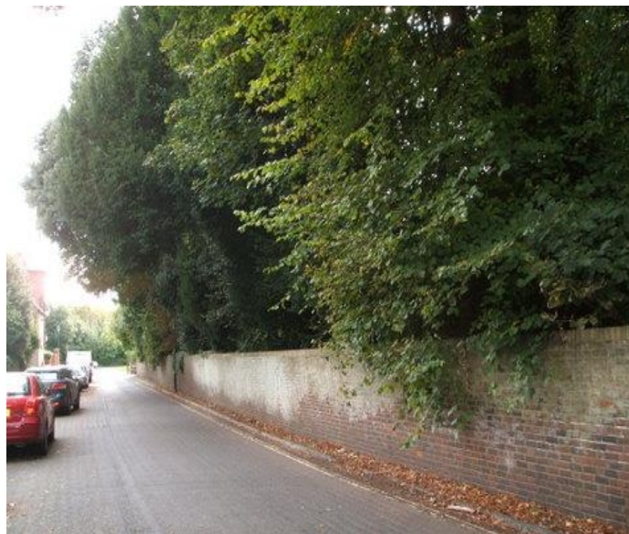
Looking south at unstable boundary wall along South Street.
