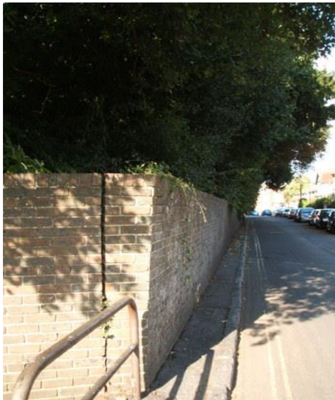
Looking north at widening gap between walls.
