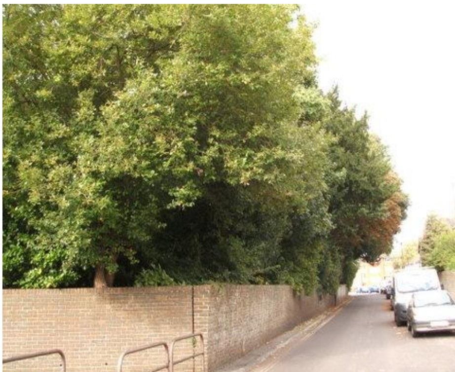
Looking north at unstable brick boundary wall with trees behind.
