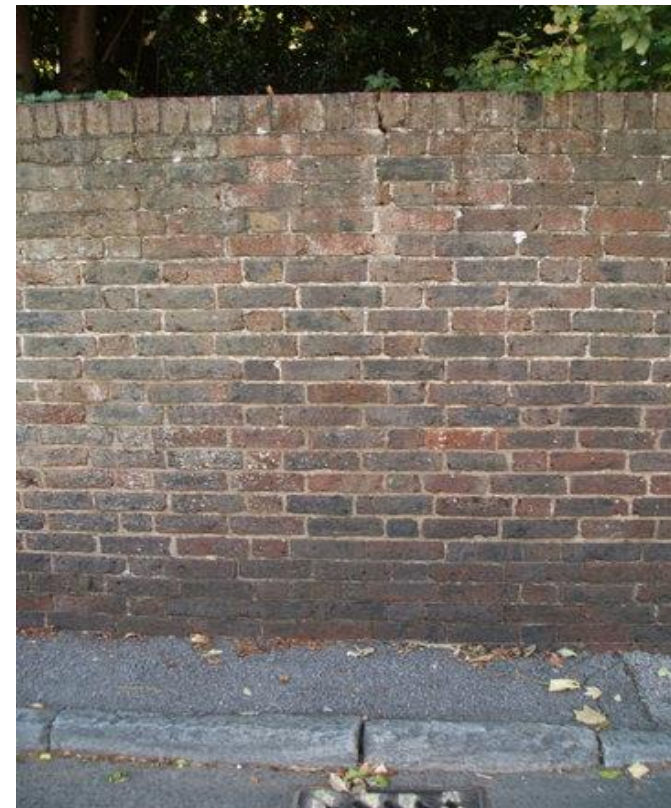
Looking west at a crack in boundary wall.
