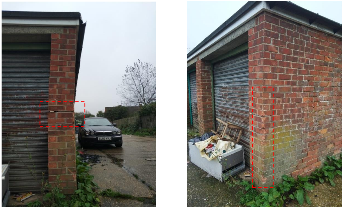
Fig. 13 – Photos showing the damaged existing garage.
