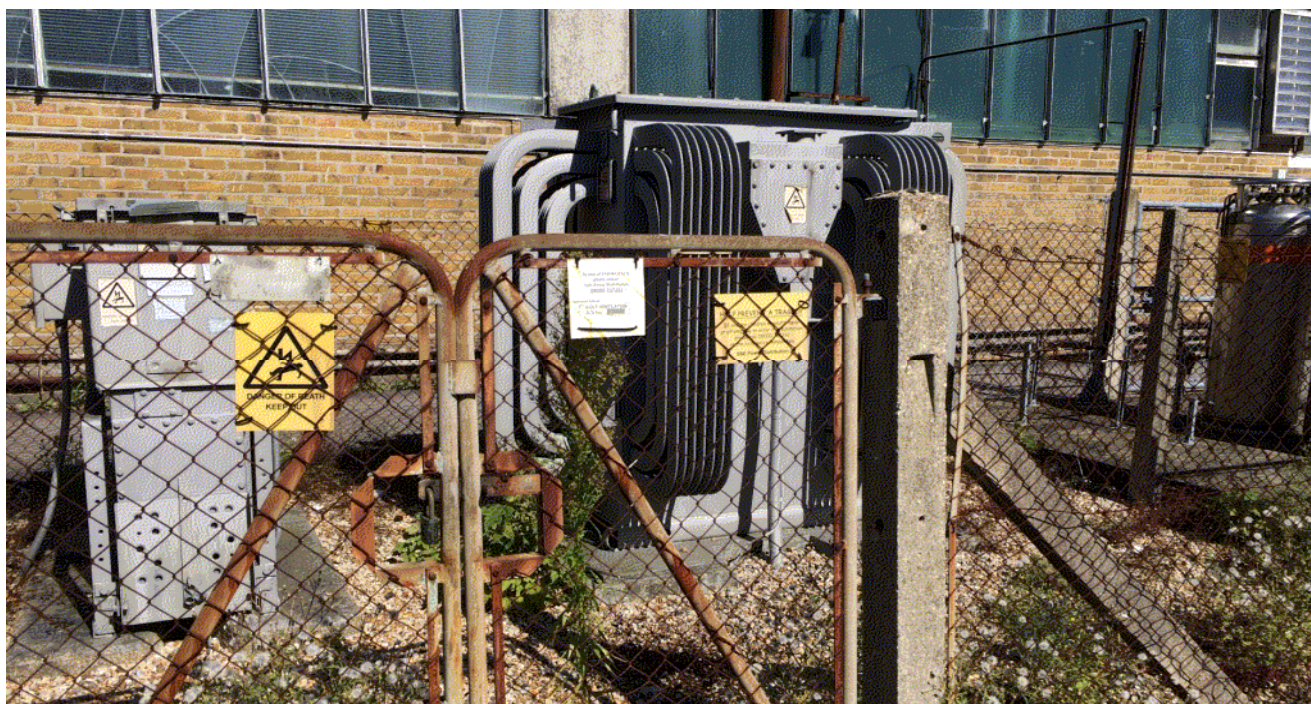
Photo 30 - Electricity Sub-Station south of main factory building
