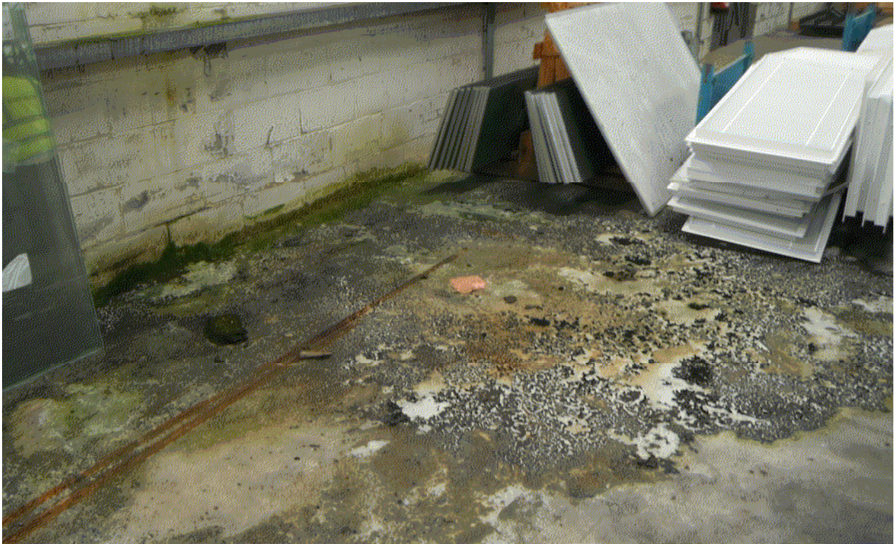
Photo 17- Lichen on floor in north west of warehouse area
