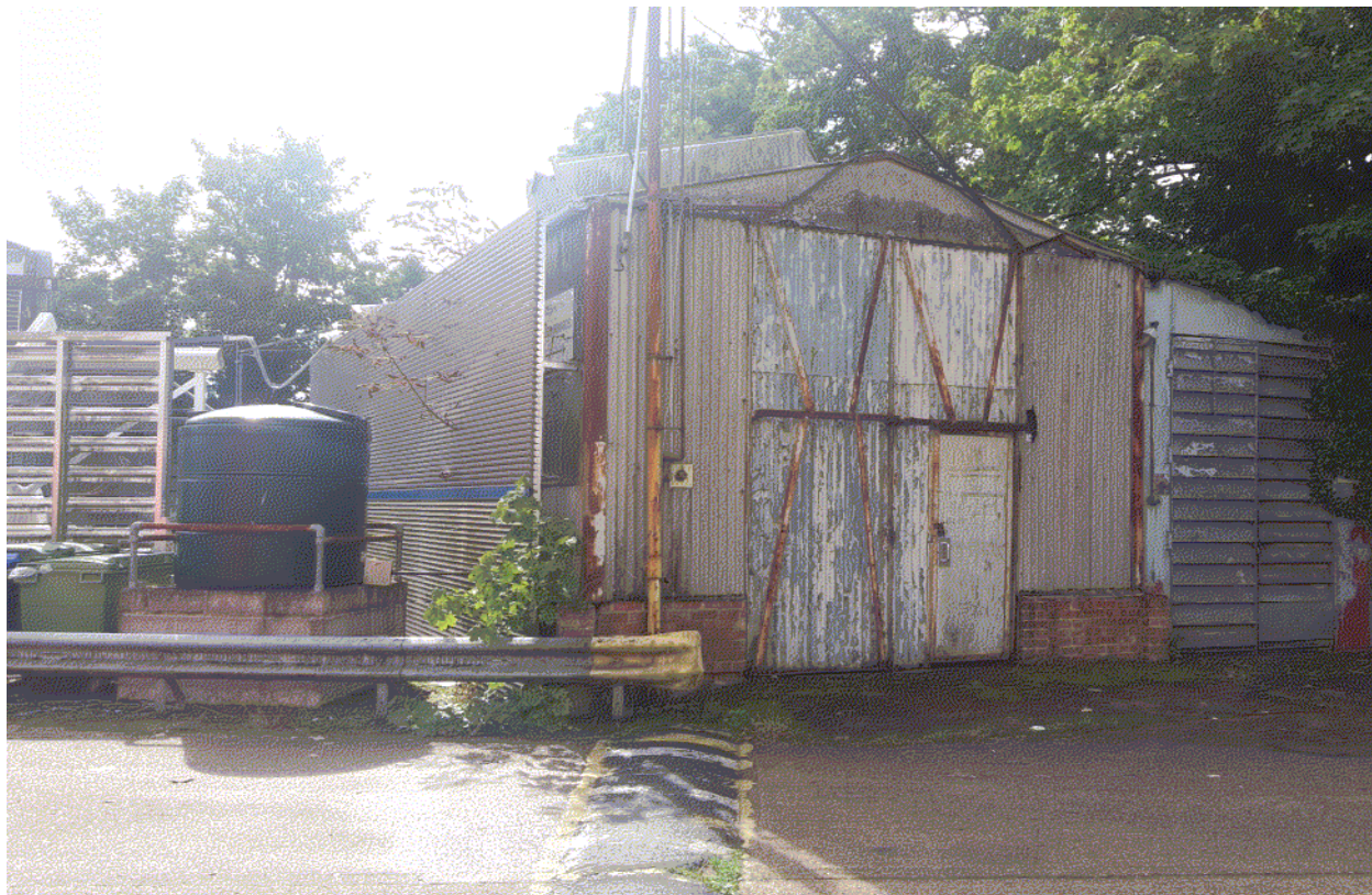
Photo 25 - Fire testing building and adjoining Fuel Oil AST in south of the site
