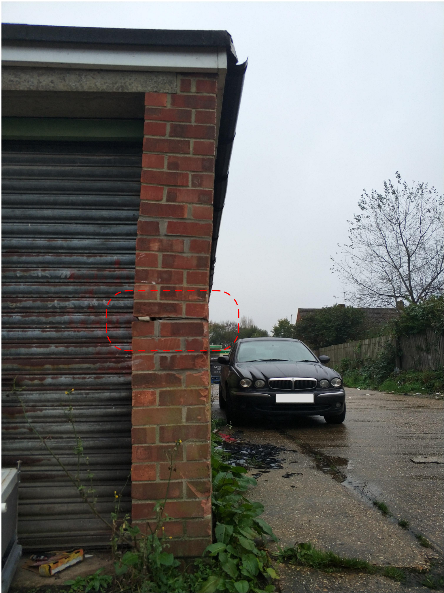
The photo is showing the damages caused by vehicle bashing to the corner of the existing garage from vehicle turning.
